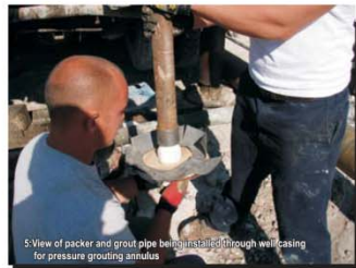
5-View of packer and grout pipe being set to through well casing for pressure grouting annulus
