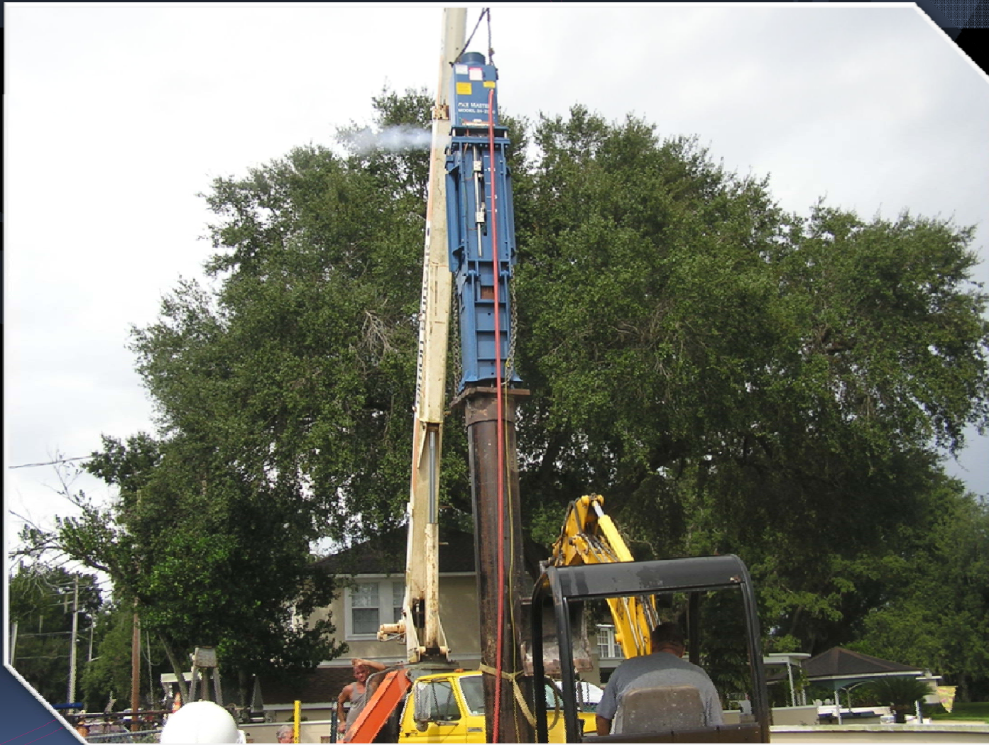
Bass Lake - View of 18-inch diameter surface casing being driven to depth using a pneumatic hammer.
