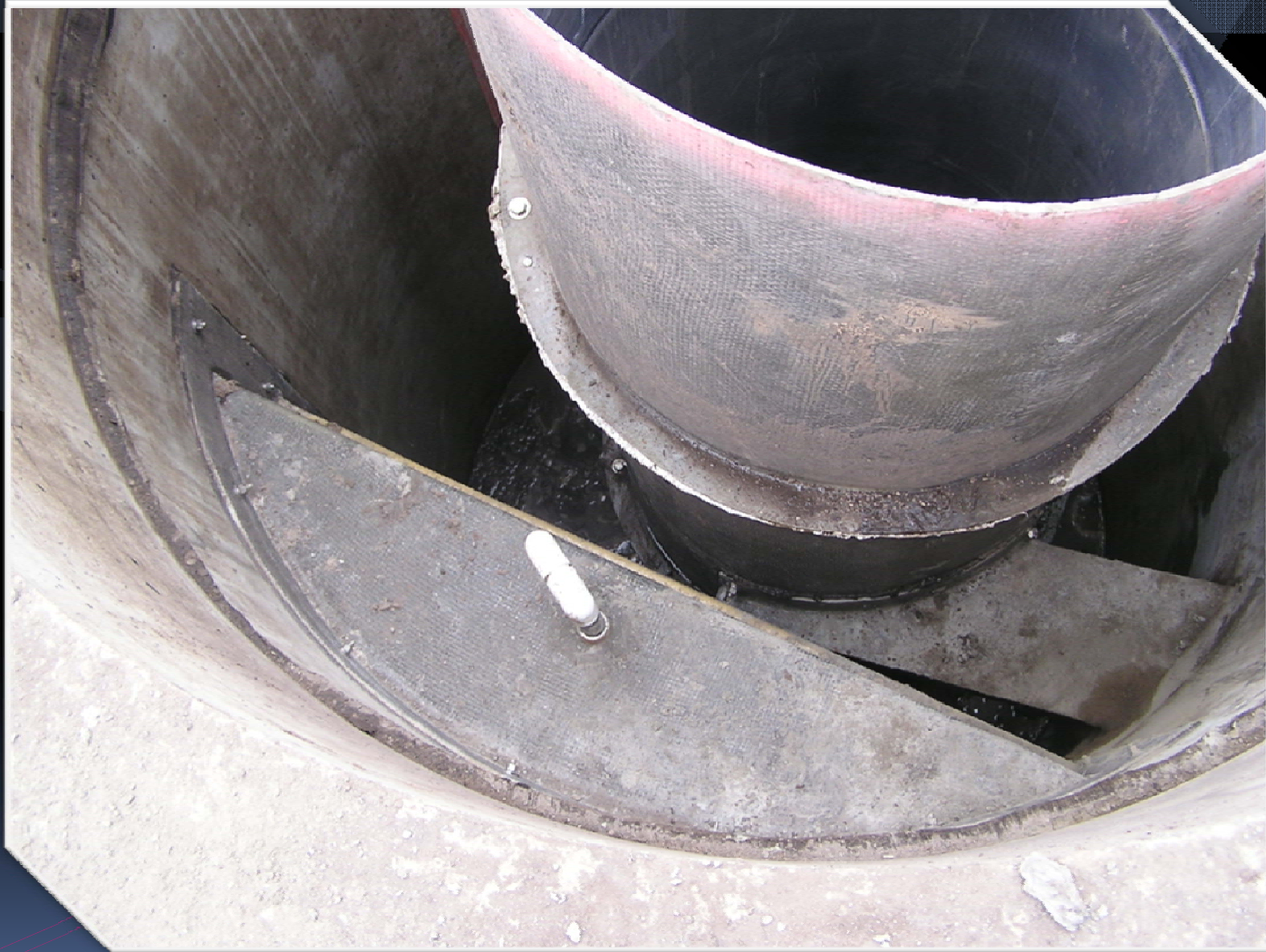
Clay Street - Oil baffle and separation screen within CDS structure.
