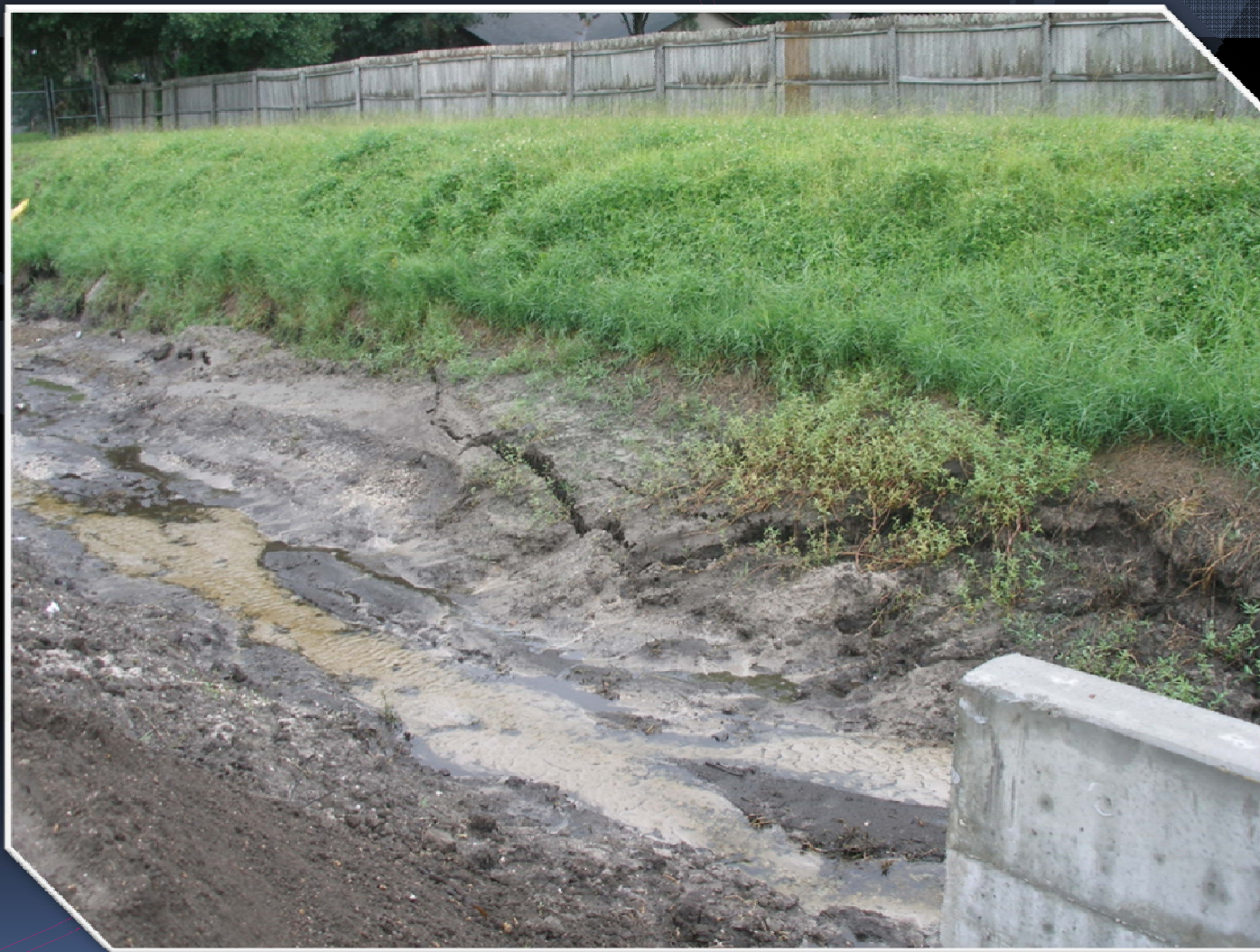
Goddard Avenue - Unstable ditch sideslope - note soil cracking.
