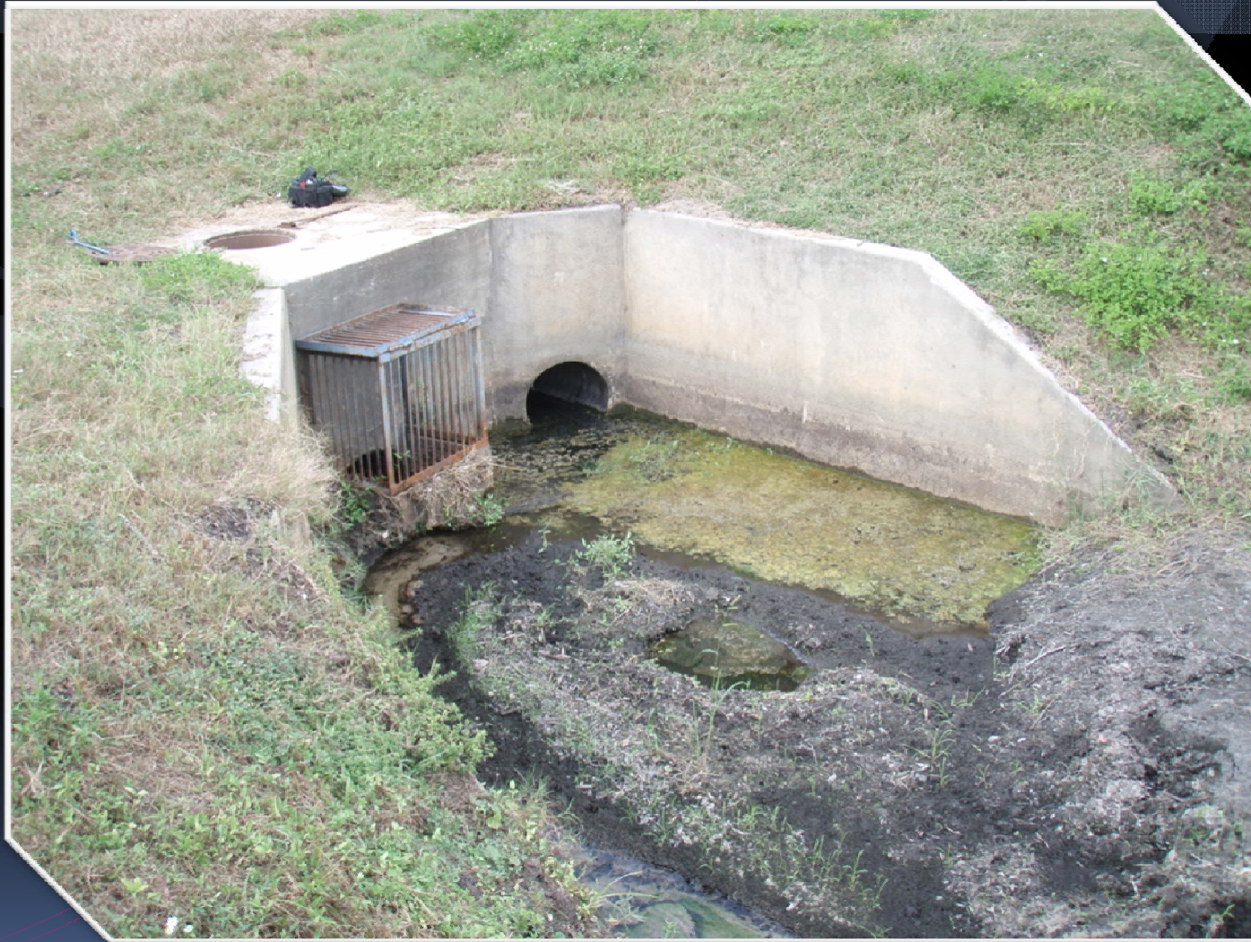
Goddard Avenue - Old headwall structure showing well intake (L) and roadway discharge (R)
