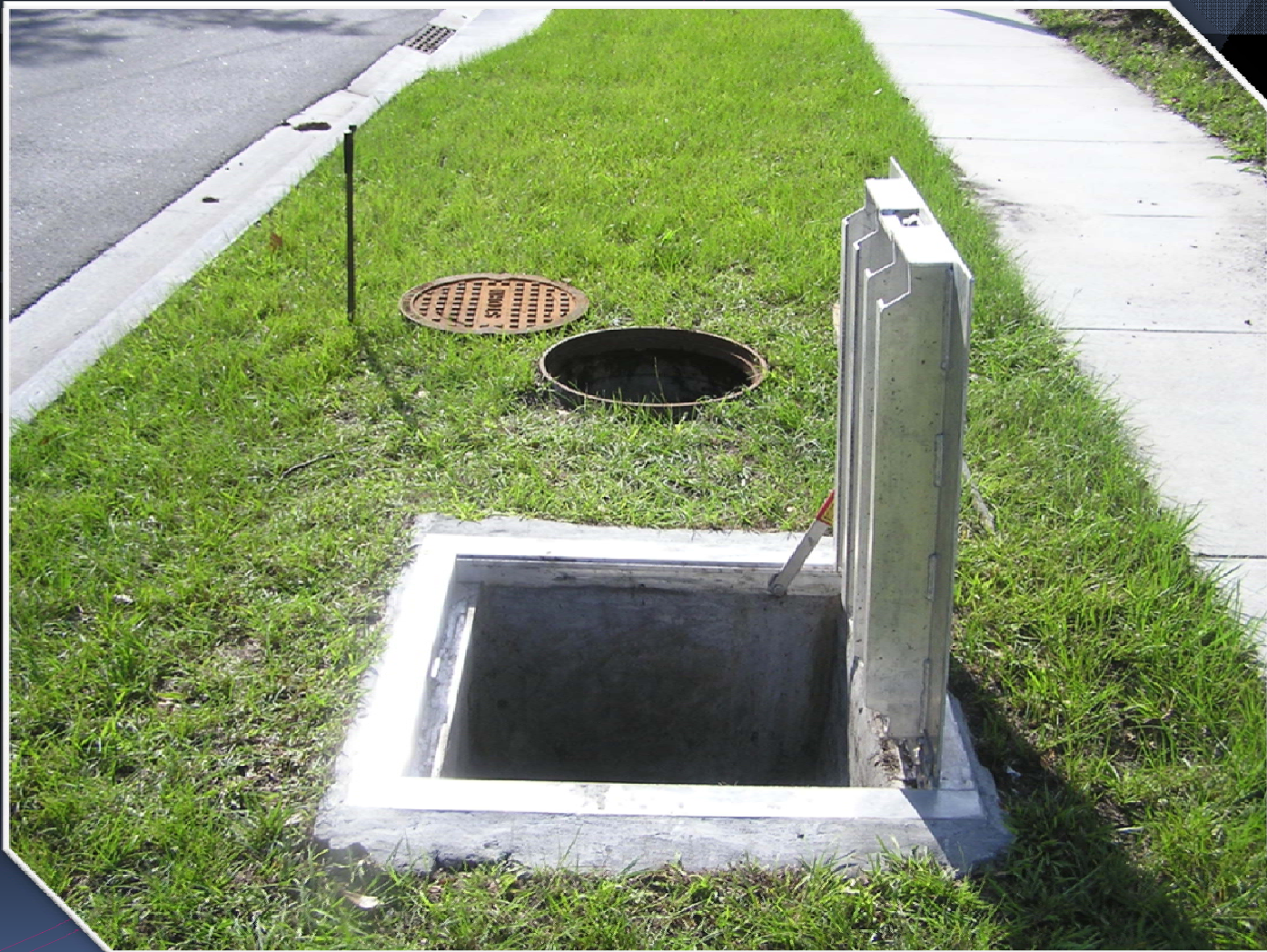
Clay Street - Access hatch and manhole cover for drainage well and weir structure.
