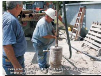
6-View of setting grout pipe at bottom of casing and sealing wellhead for pressure grouting
