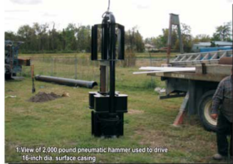
1-View of 2,000 pound pneumatic hammer used to drive 16-inch dia. surface casing
