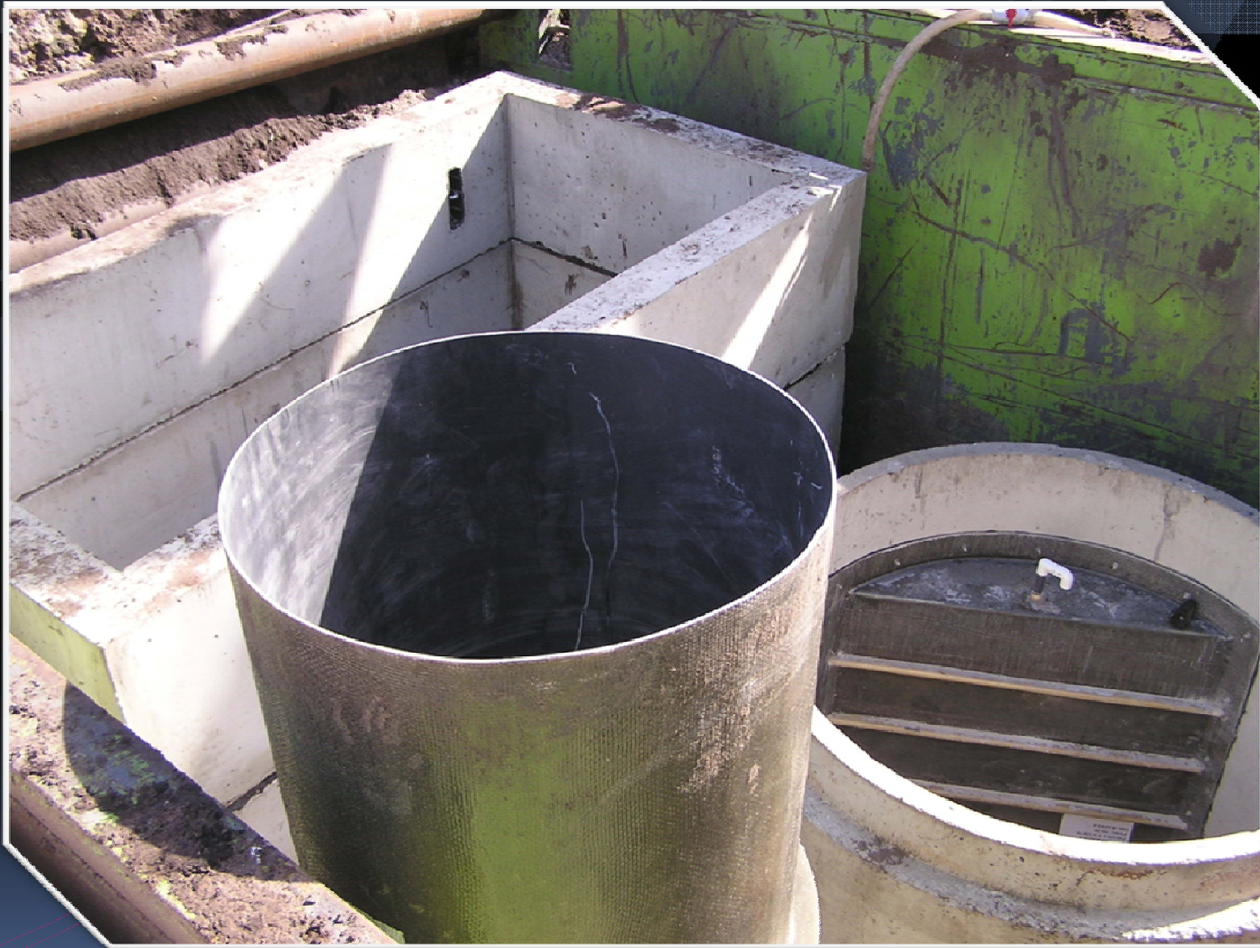
Clay Street - Additional view of CDS and drainage well structures.
