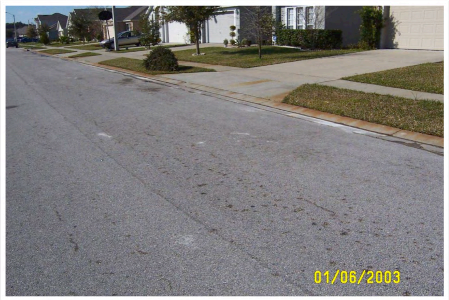
Leaching Over Curb
