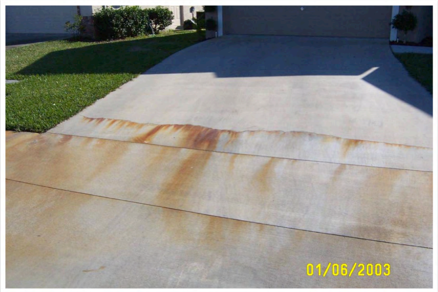
Leaching Over Curb
