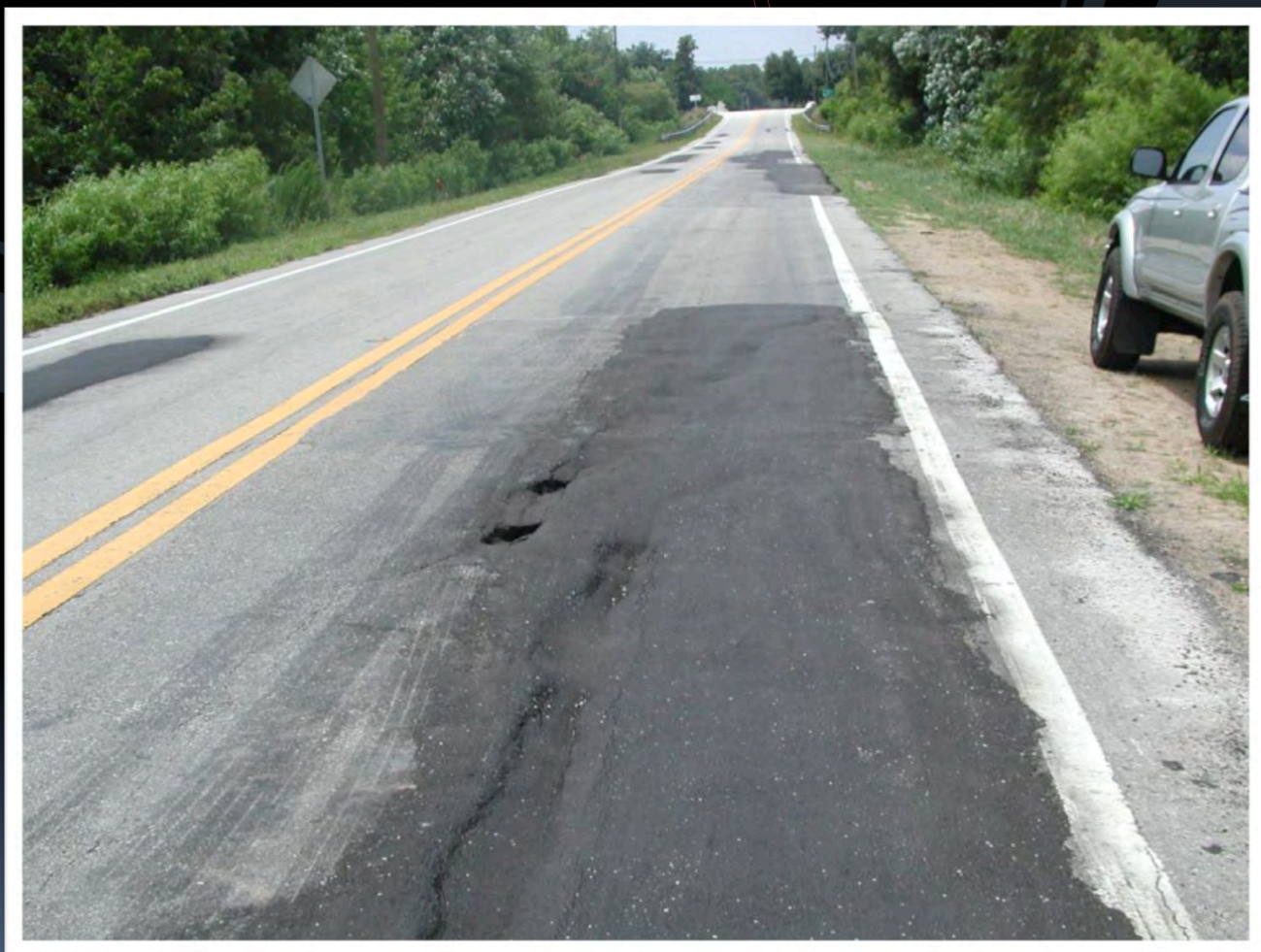
Continued pavement distress after patch
