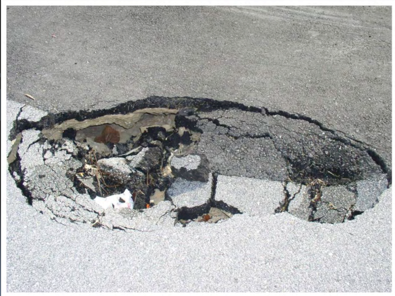
Close-up view of "sinkhole"
