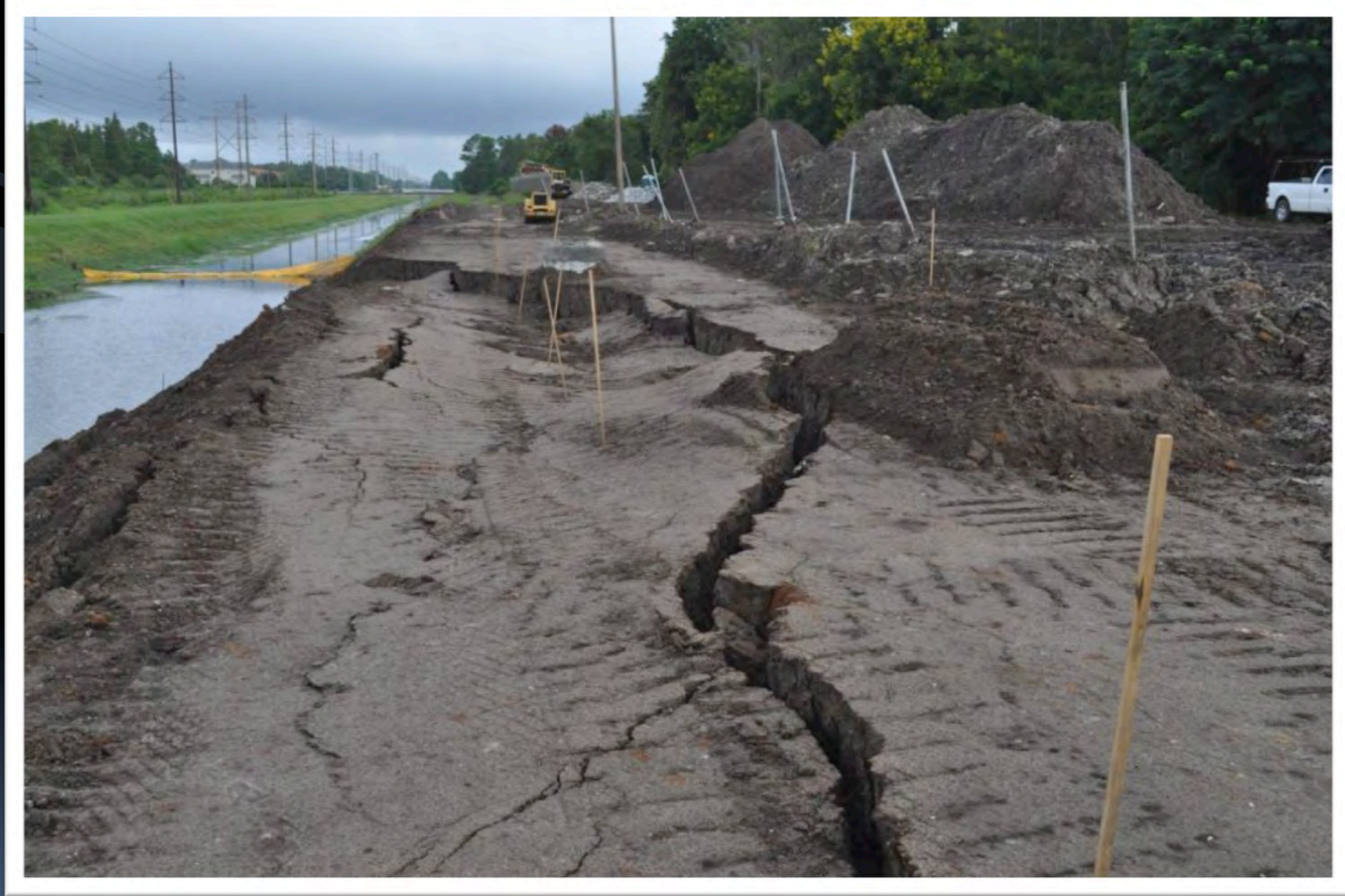
Failure of filled slope due to improper locking
