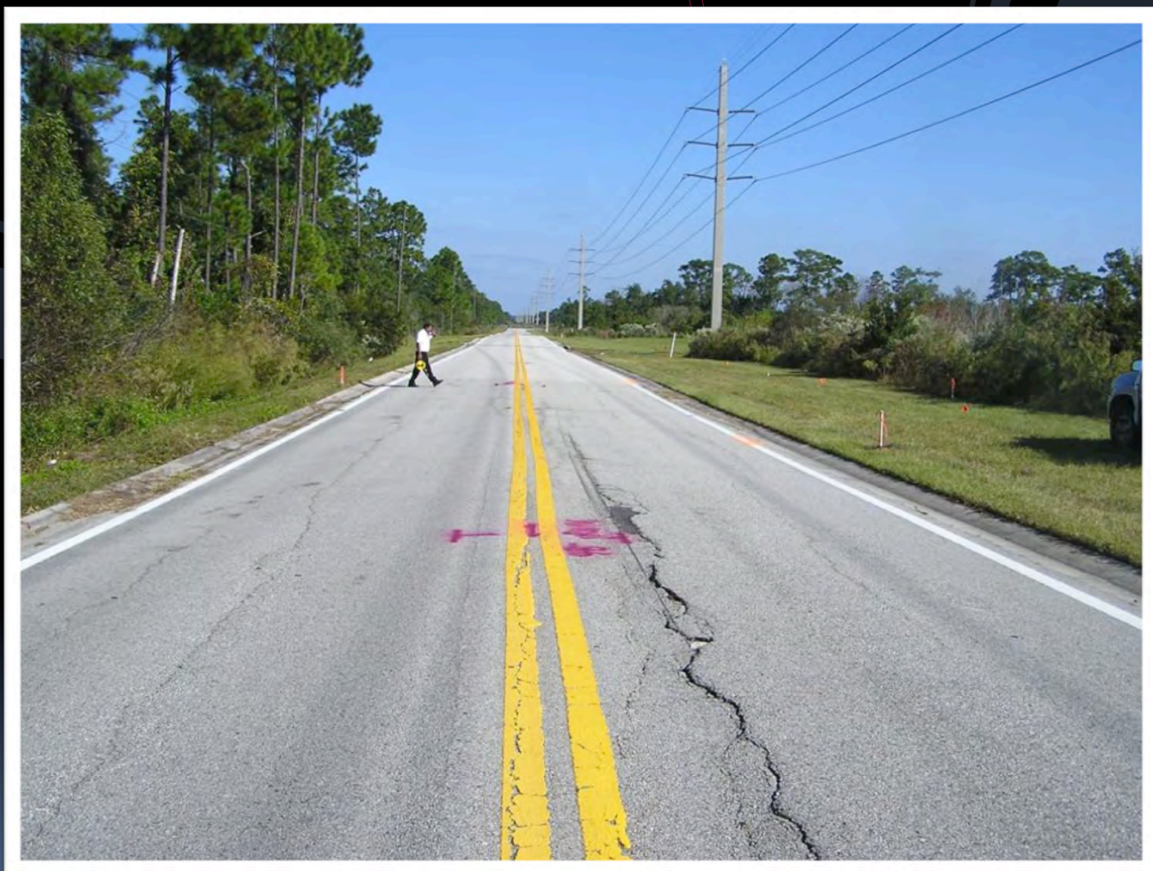
Photos of Distress
