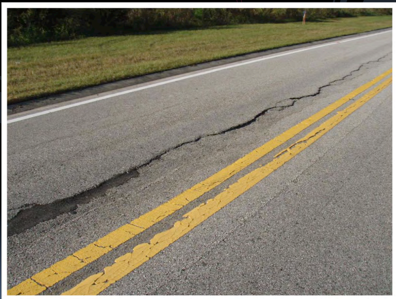
Photos of Distress
