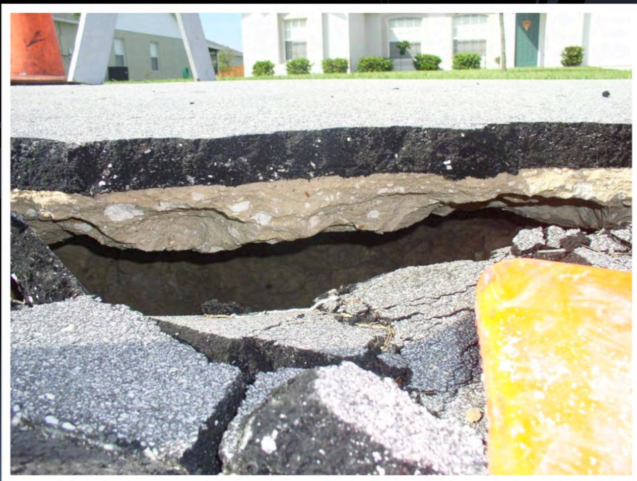
Close-up view of "sinkhole"
