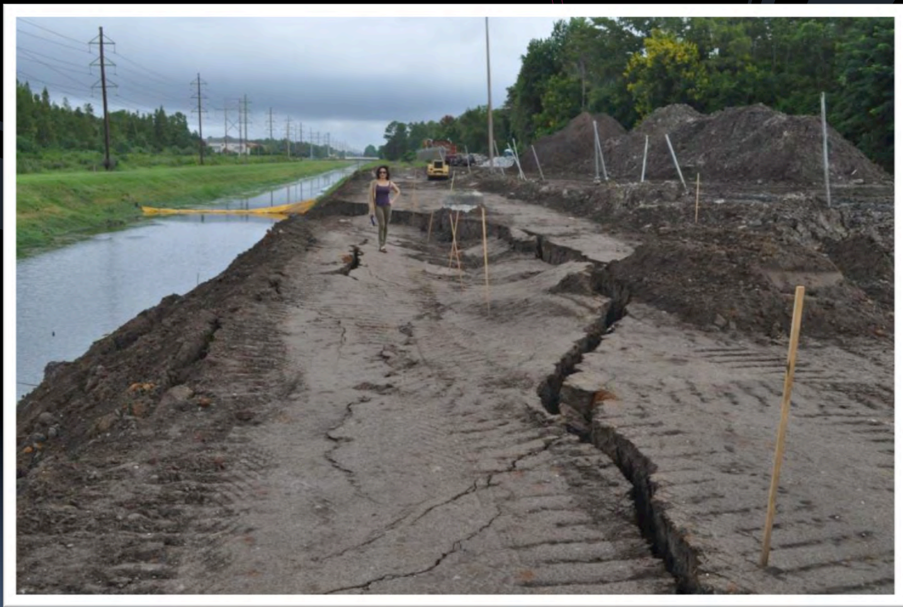
Failure due to pretty surcharge load
