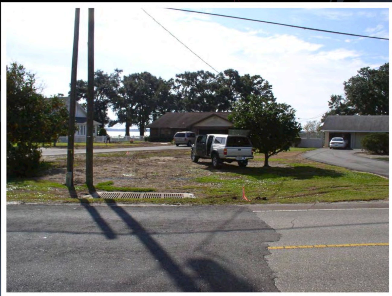
Loss of soil & settlement distress at pipe crossing
