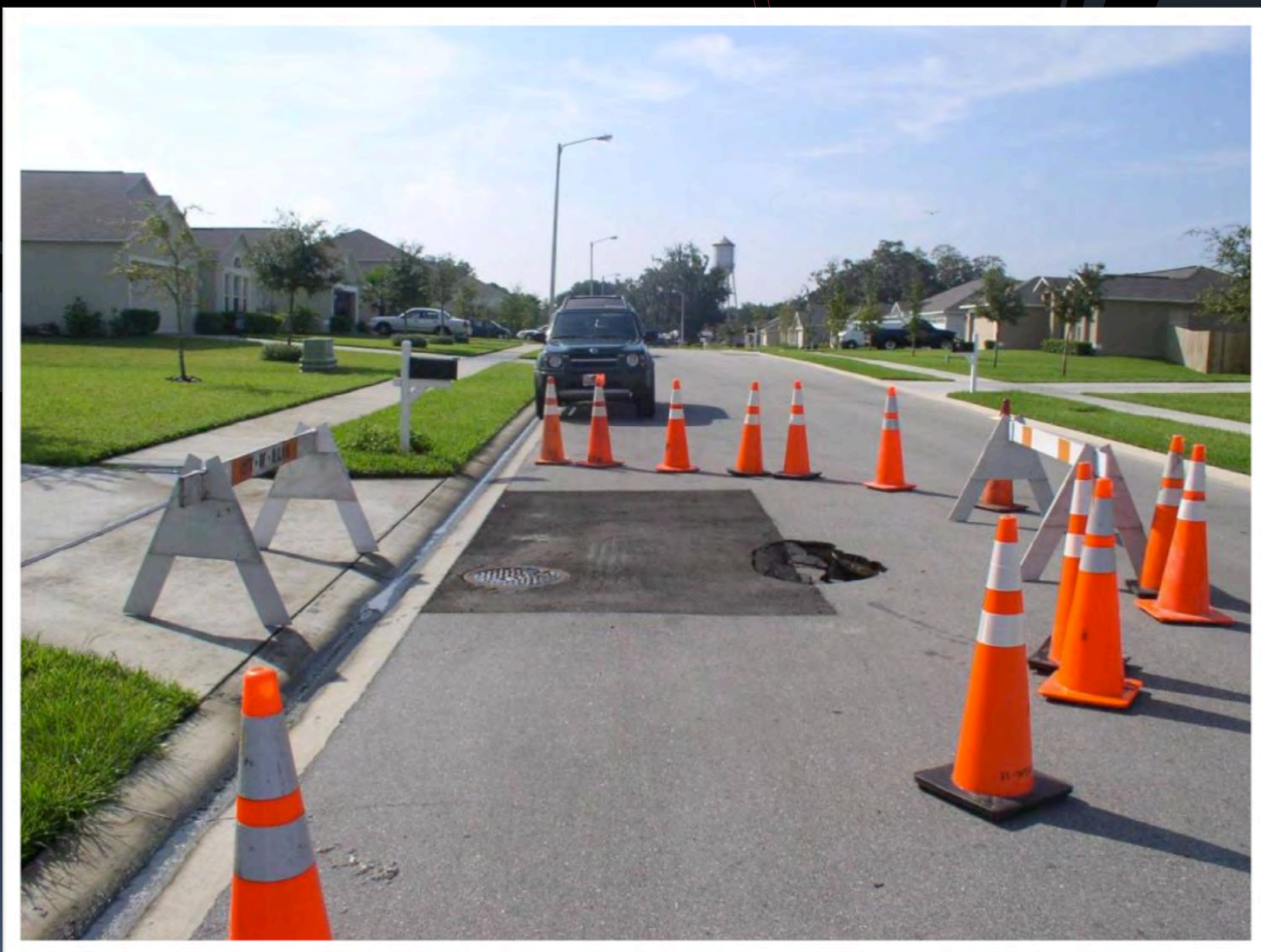
Sand flowing into leaking manhole leading to loss of soil and "sinkhole"
