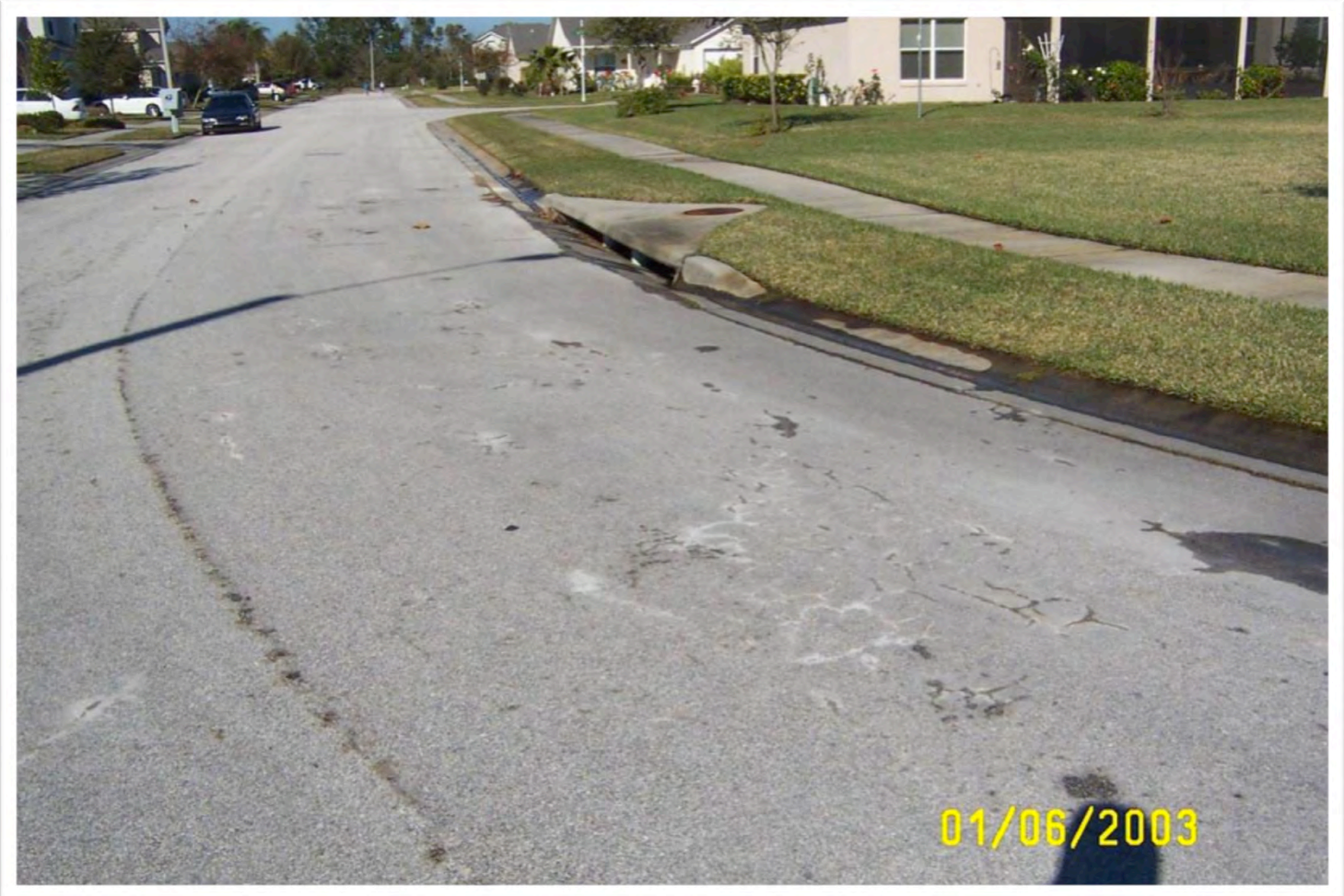
Leaching Over Curb
