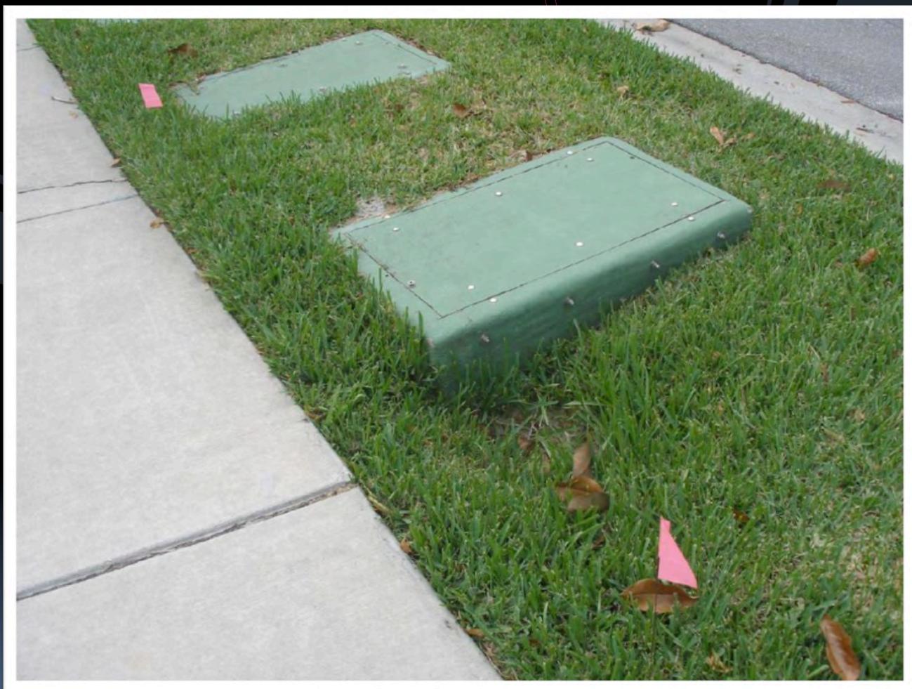
Settlement of soil around structure
