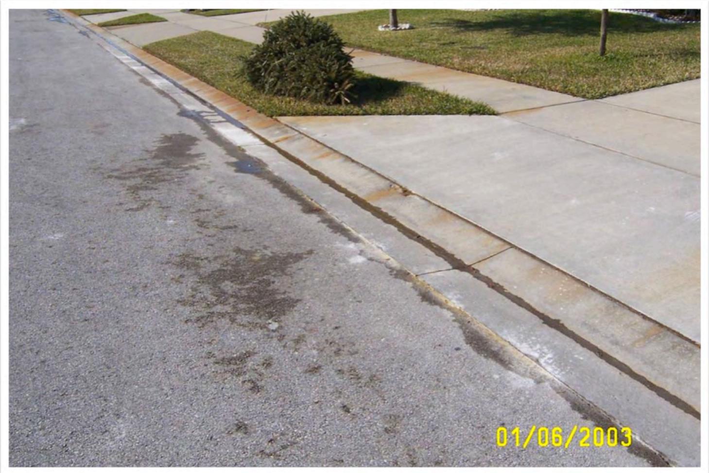
Leaching Over Curb
