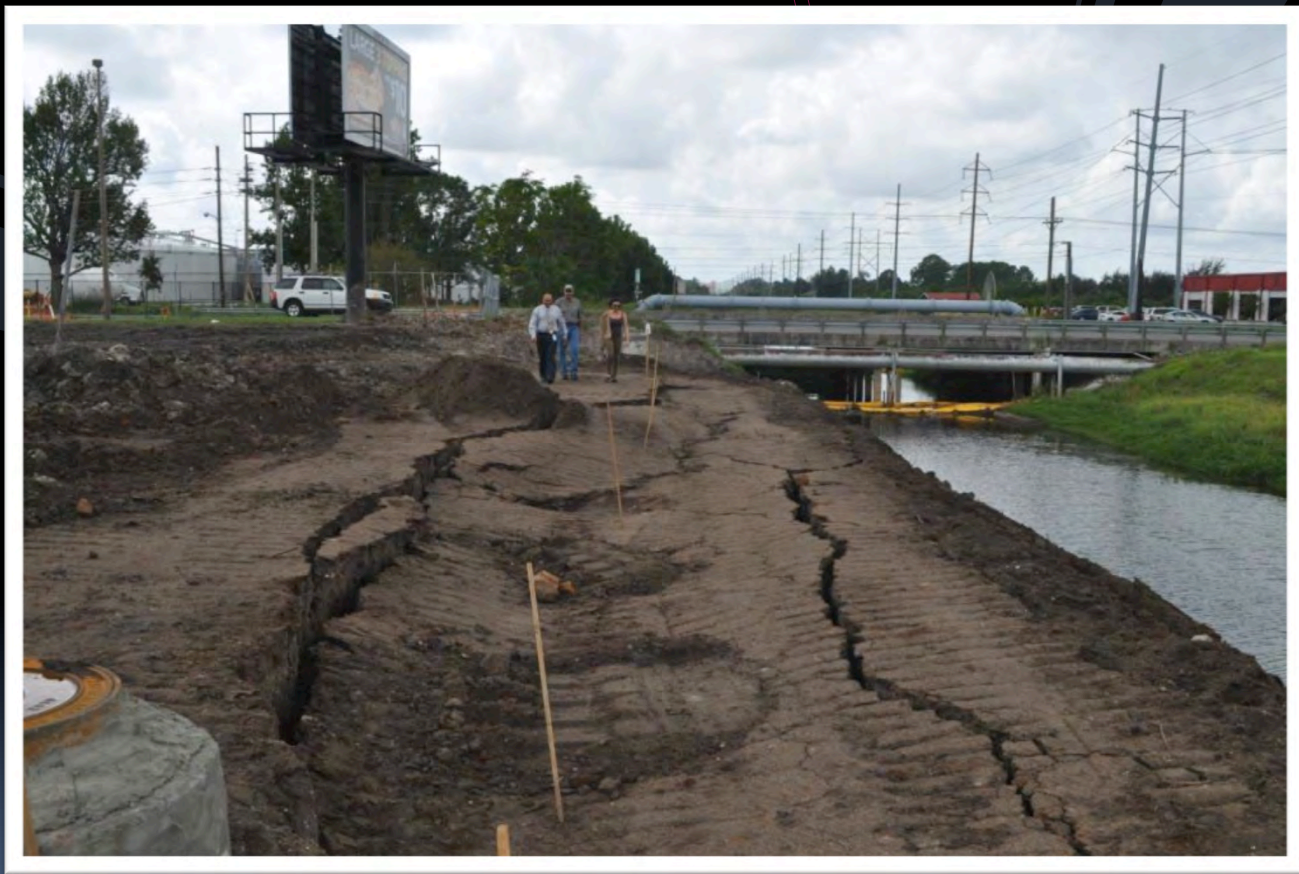
Another view of failed slope
