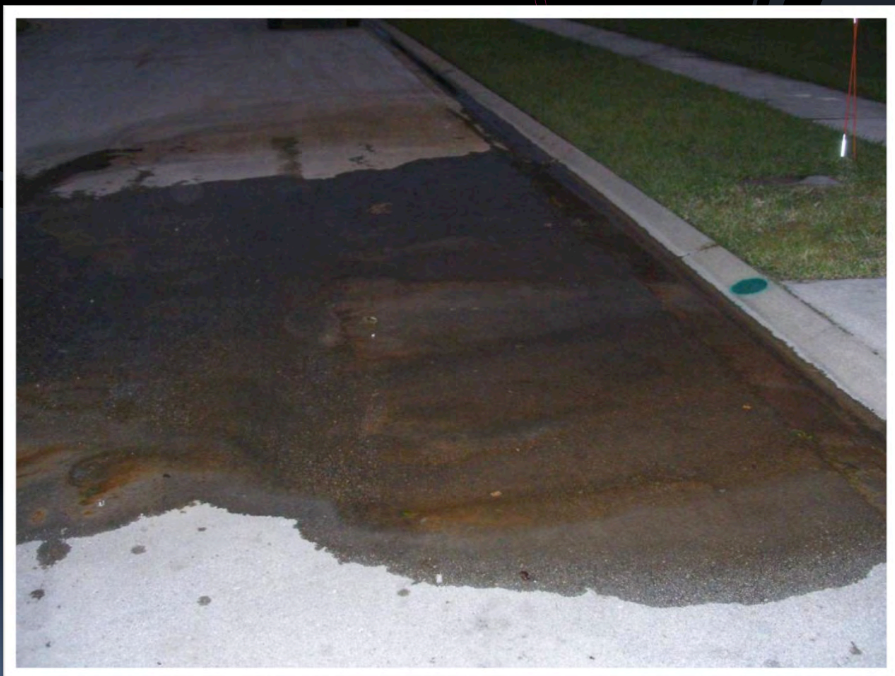
Upward Seepage Beneath Pavement
