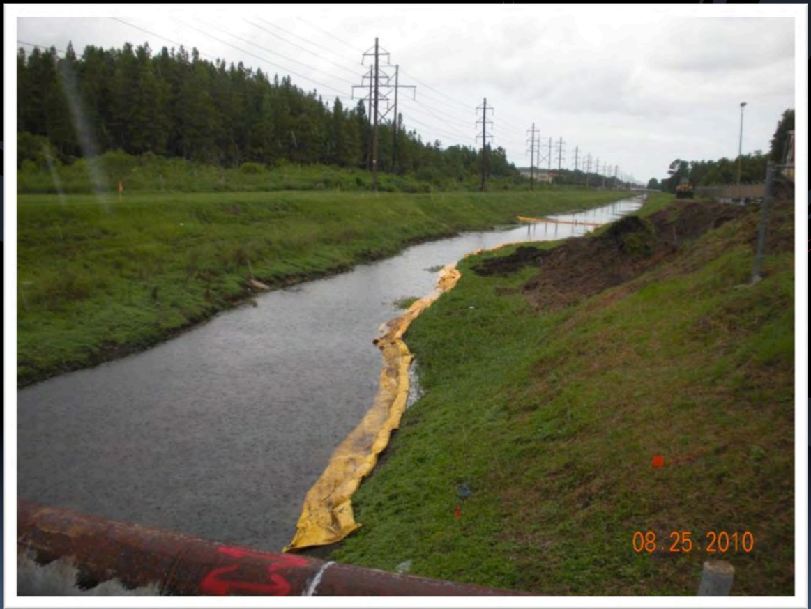
View of slope failure before any attempt to reshape
