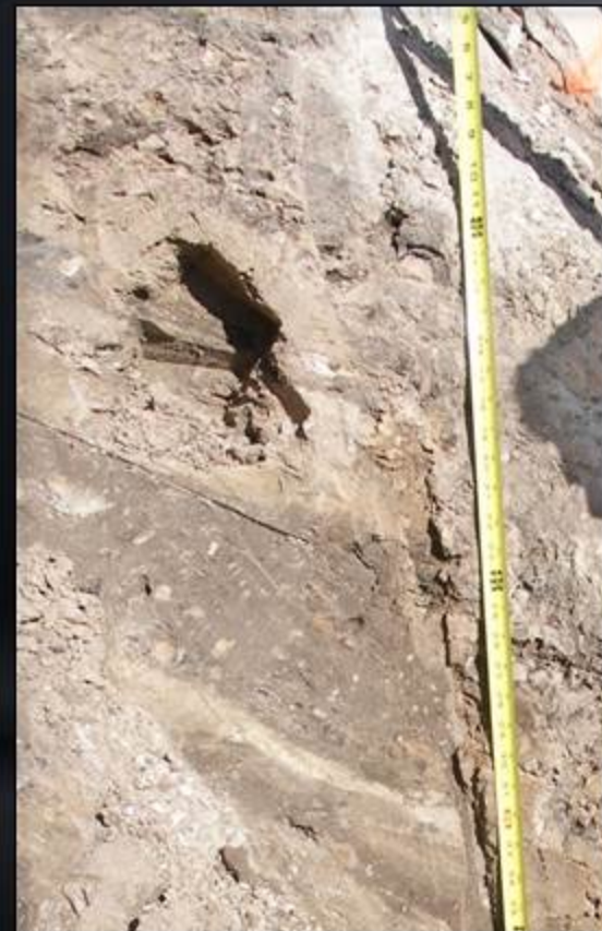
Close-up view of the shear failure plane on the northern pit wall
