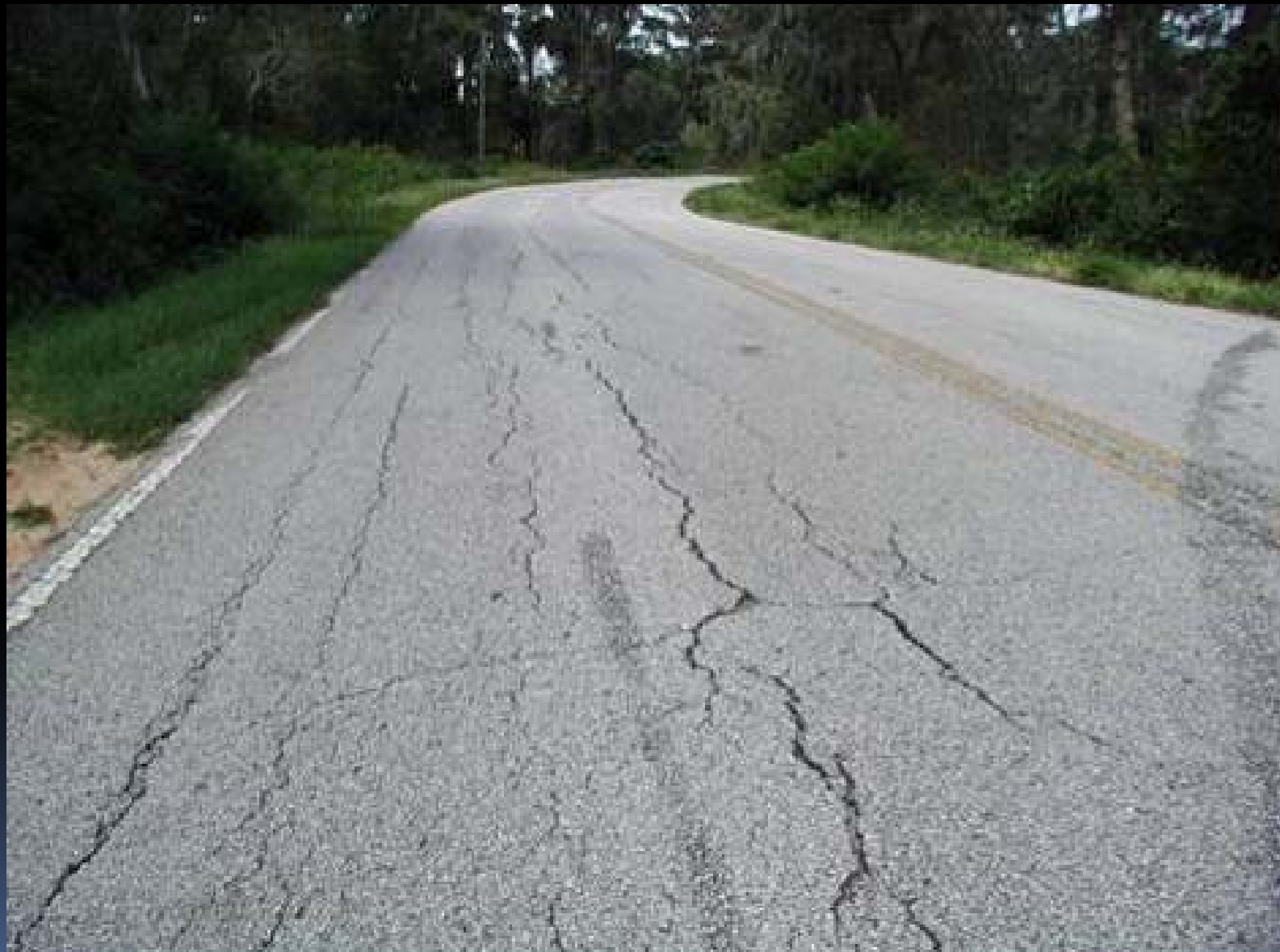
Pavement Distress Due To Buried Peat
