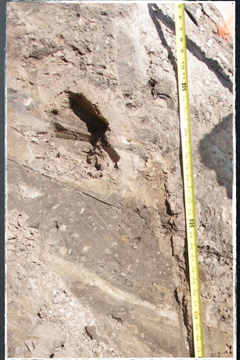
Close-up view of the shear failure plane on the northern pit wall
