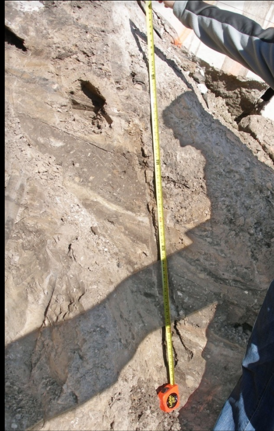
View looking at the shear failure plane on the northern pit wall
