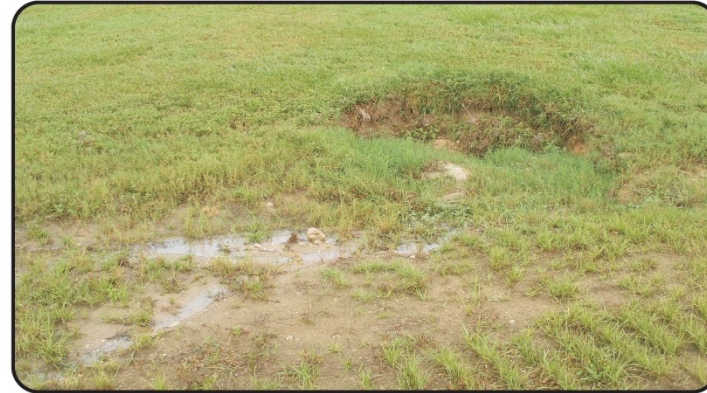
Photo 2. Shows Water Flowing Into The Sinkhole at the Toe of Slope on the Western Side of Pond SMF-1 on October 24, 2007
