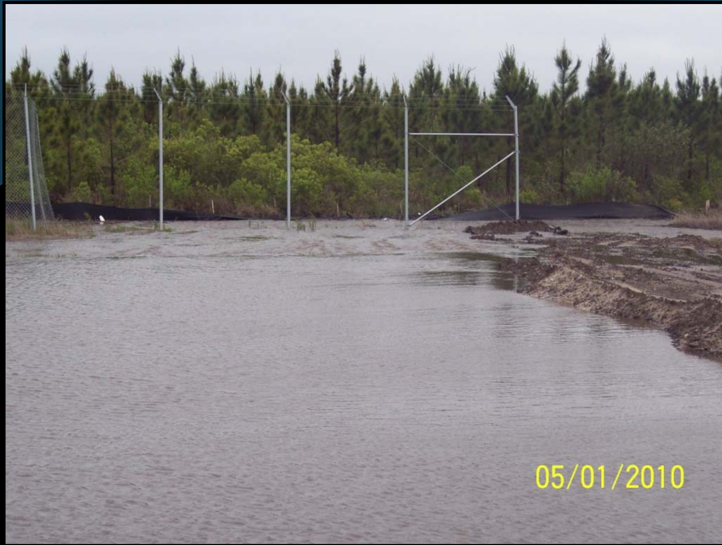
Obstruction of Natural Drainage Flow Path During Construction
