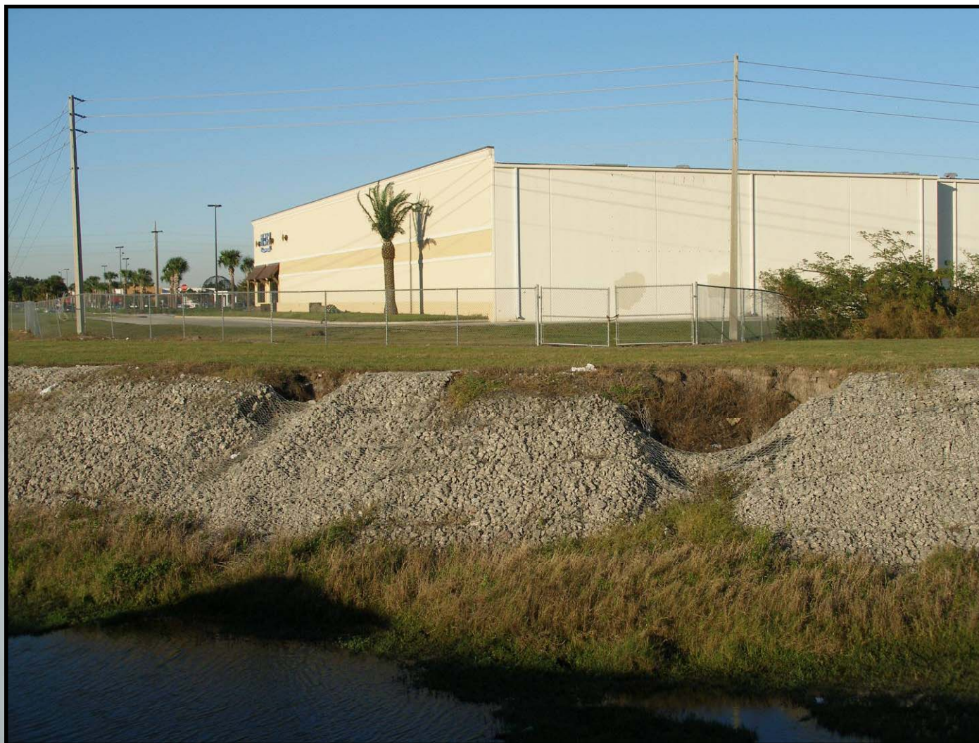
Movement of reno mattress on steep canal slope
