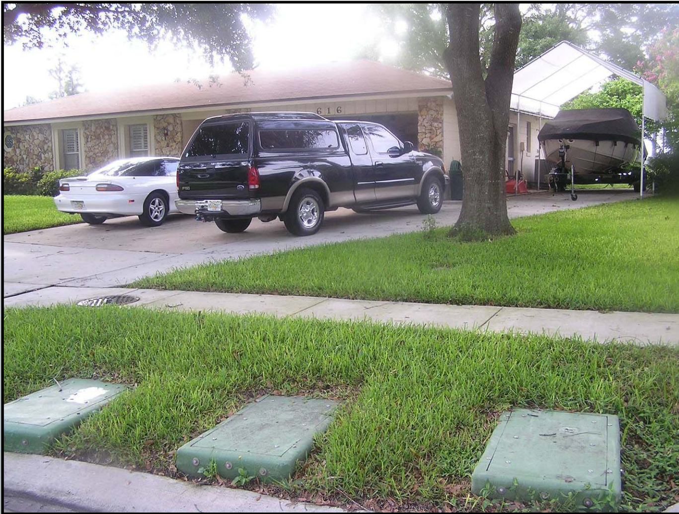
Installed structure in landscape strip
