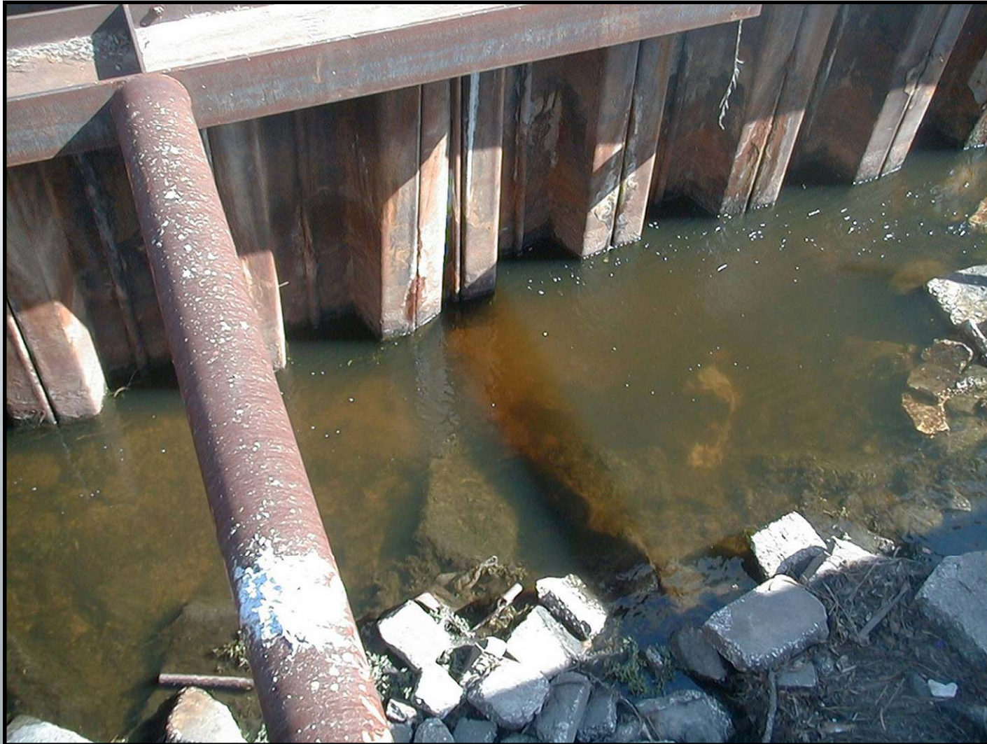
Grout loss directly below angled sheet piles
