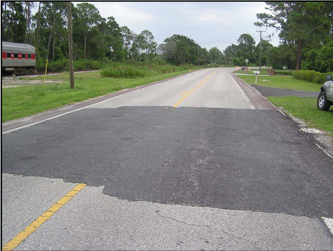
Pavement reinstated after settlement
