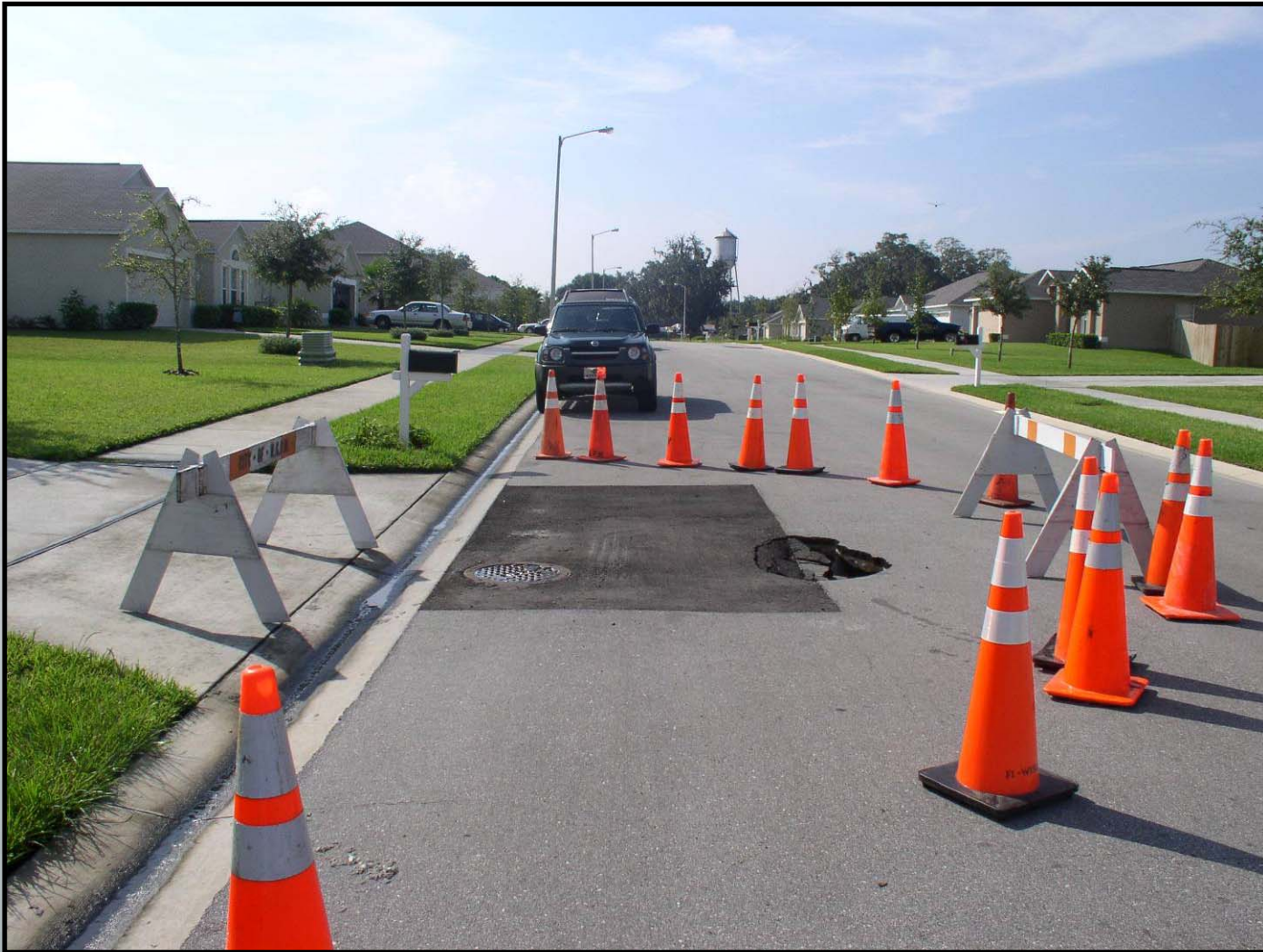
Sand flowing into leaking manhole leading to loss of soil and "sinkhole"
