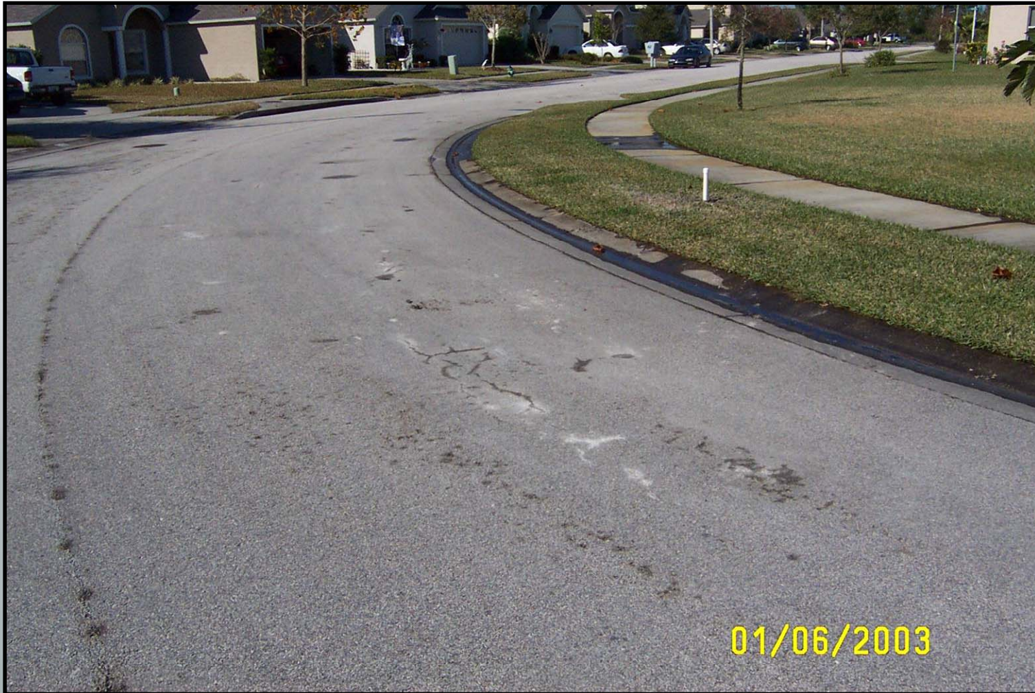
Leaching Over Curb
