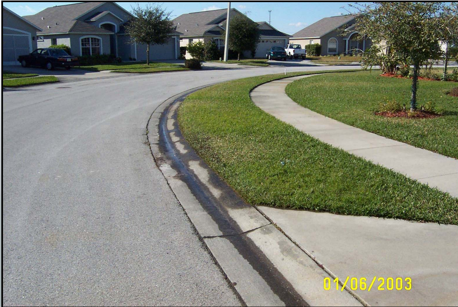
Leaching Over Curb
