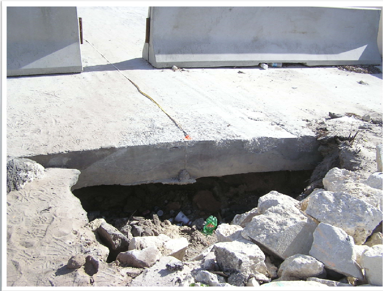
REUNION BRIDGE- Initiation of Underscour of the Approach Slab
