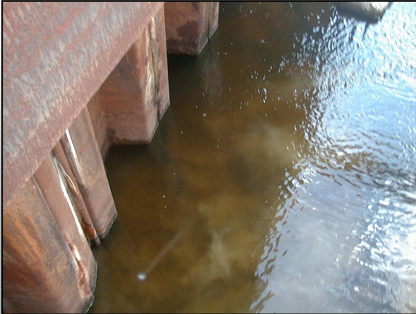
Close-up view of grout loss
