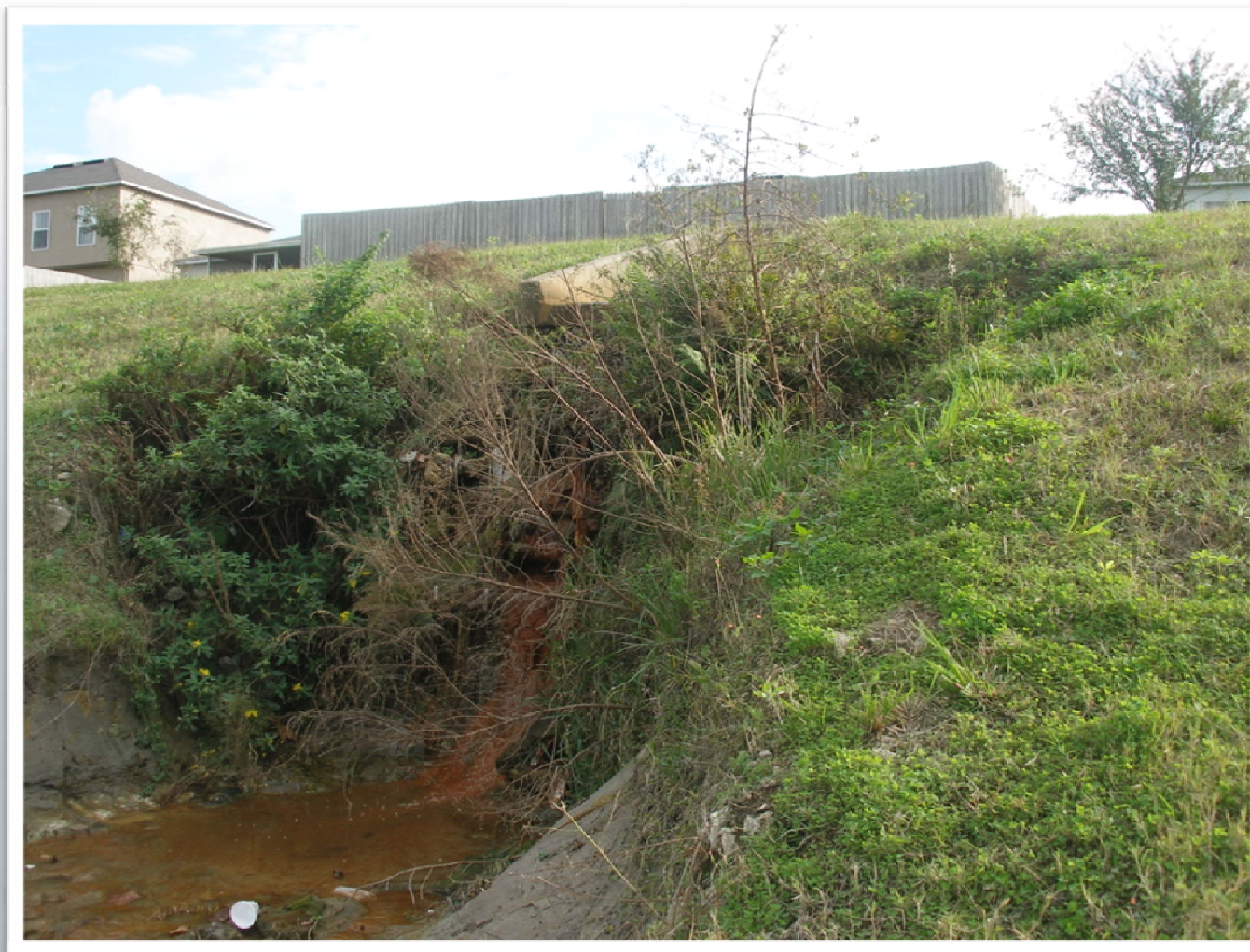
WESTLAKE-Scour And Erosion @ Storm Inlet to Pond
