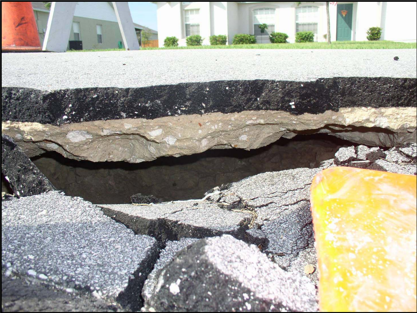
Close-up view of “sinkhole”
