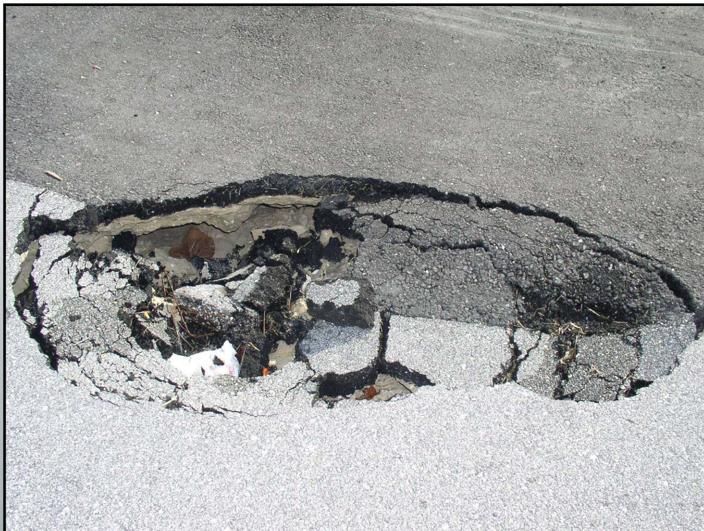
Close-up view of "sinkhole"
