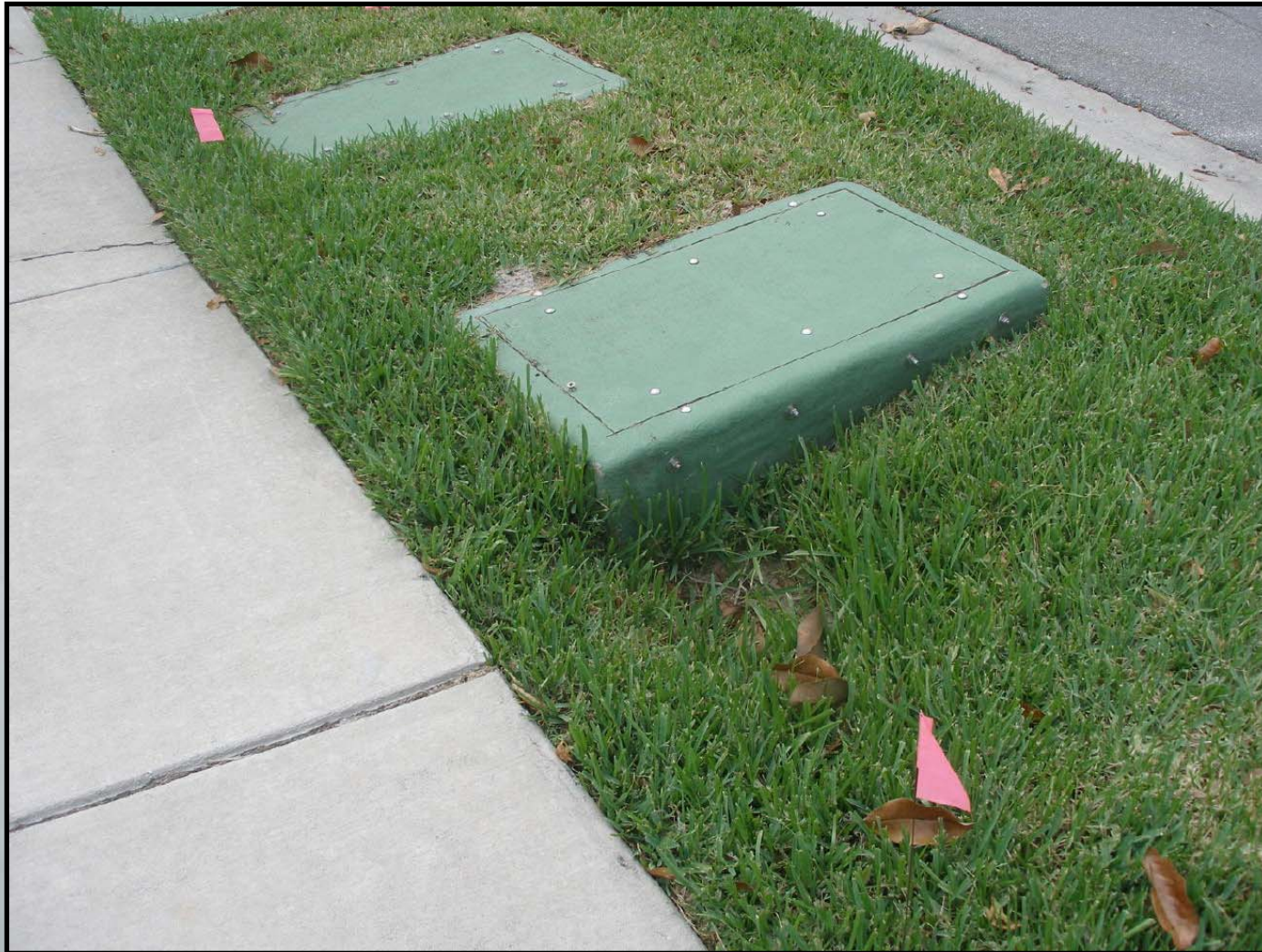
Settlement of soil around structure
