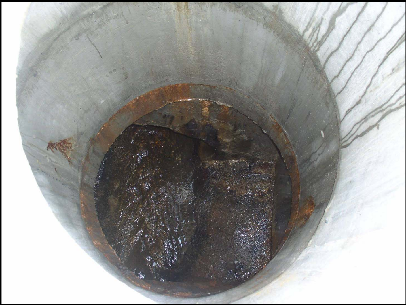
Interior view of leaking manhole
