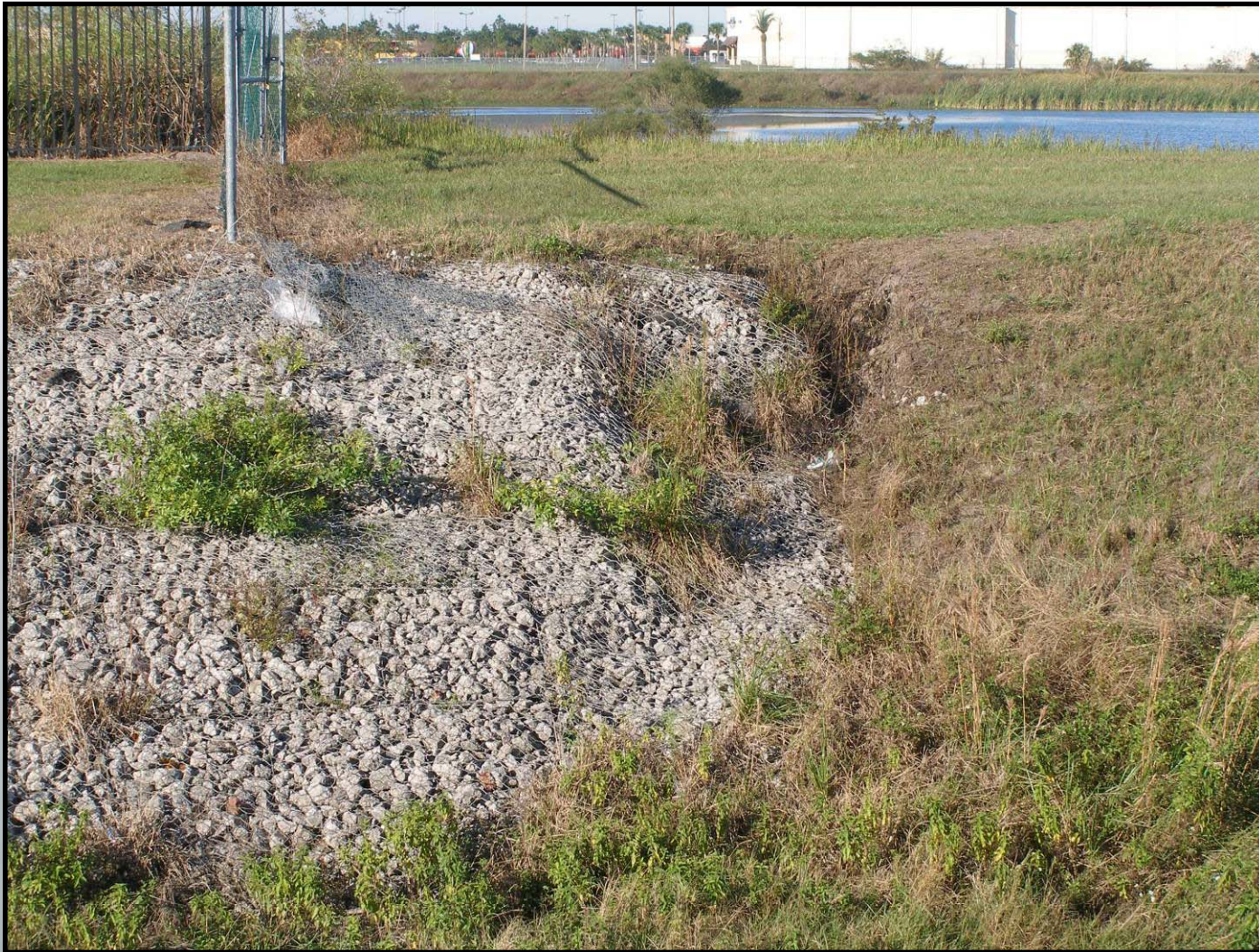
Slippage of reno mattress due to lack of anchorage on steep slope
