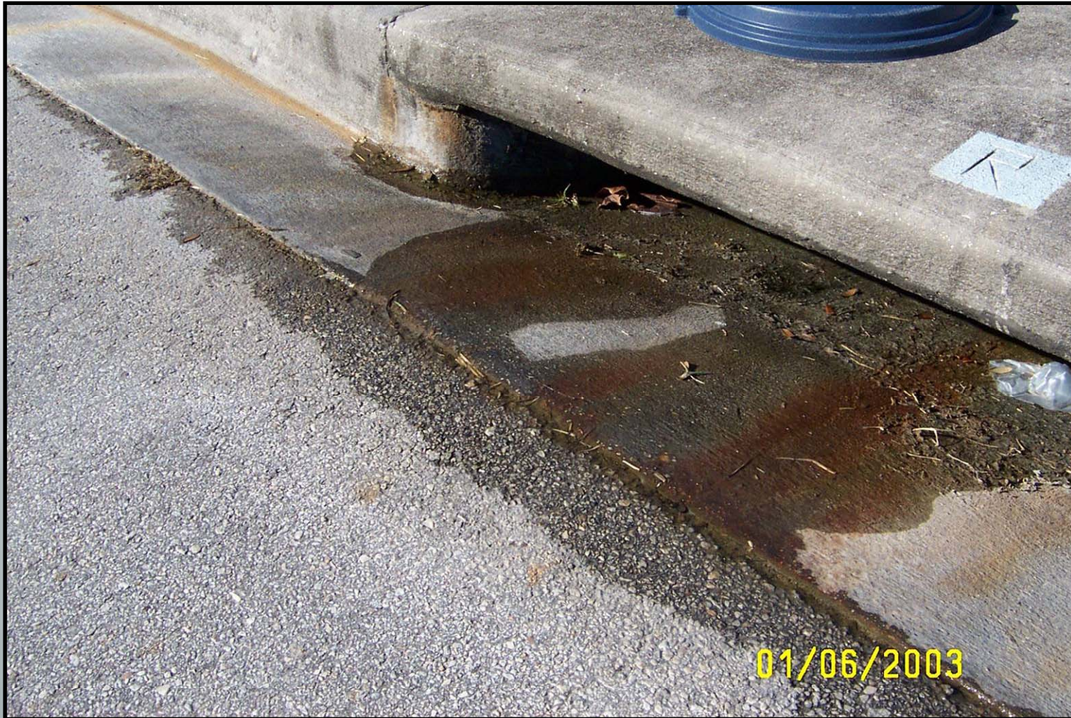
Leaching Over Curb
