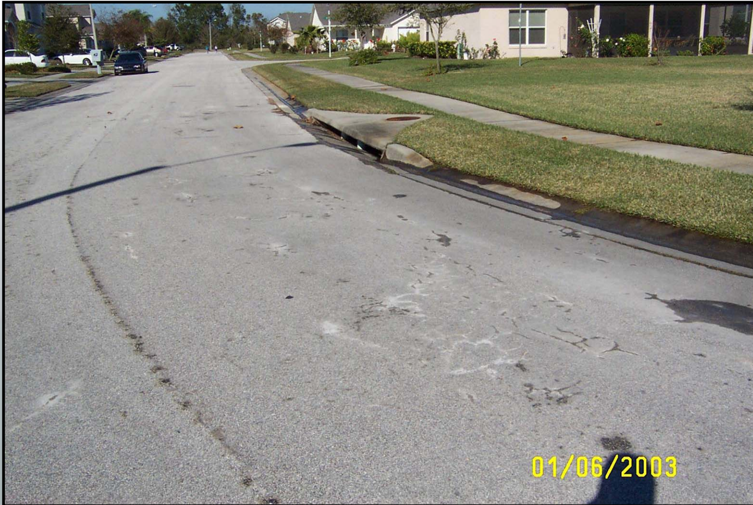
Leaching Over Curb
