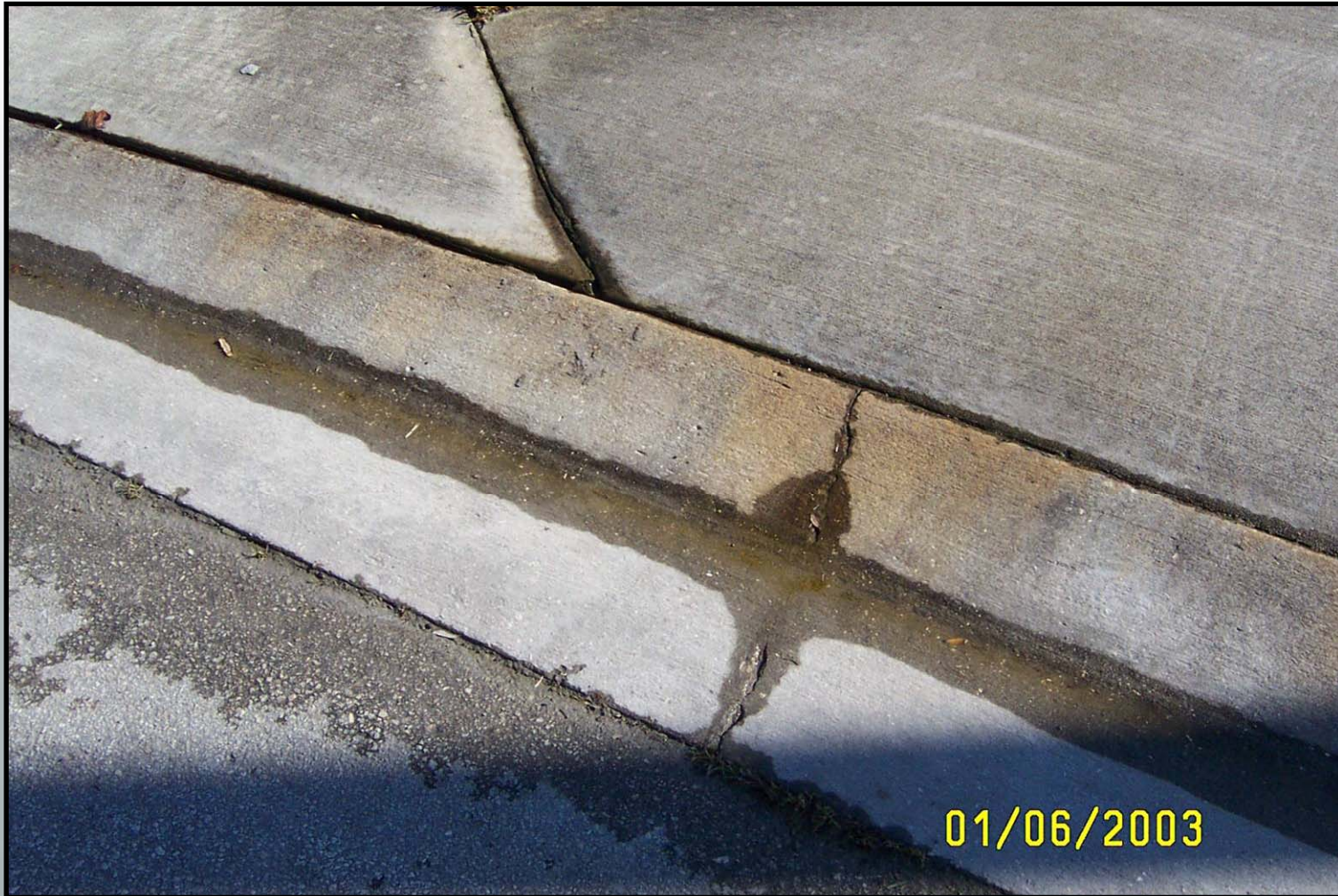
Leaching Over Curb
