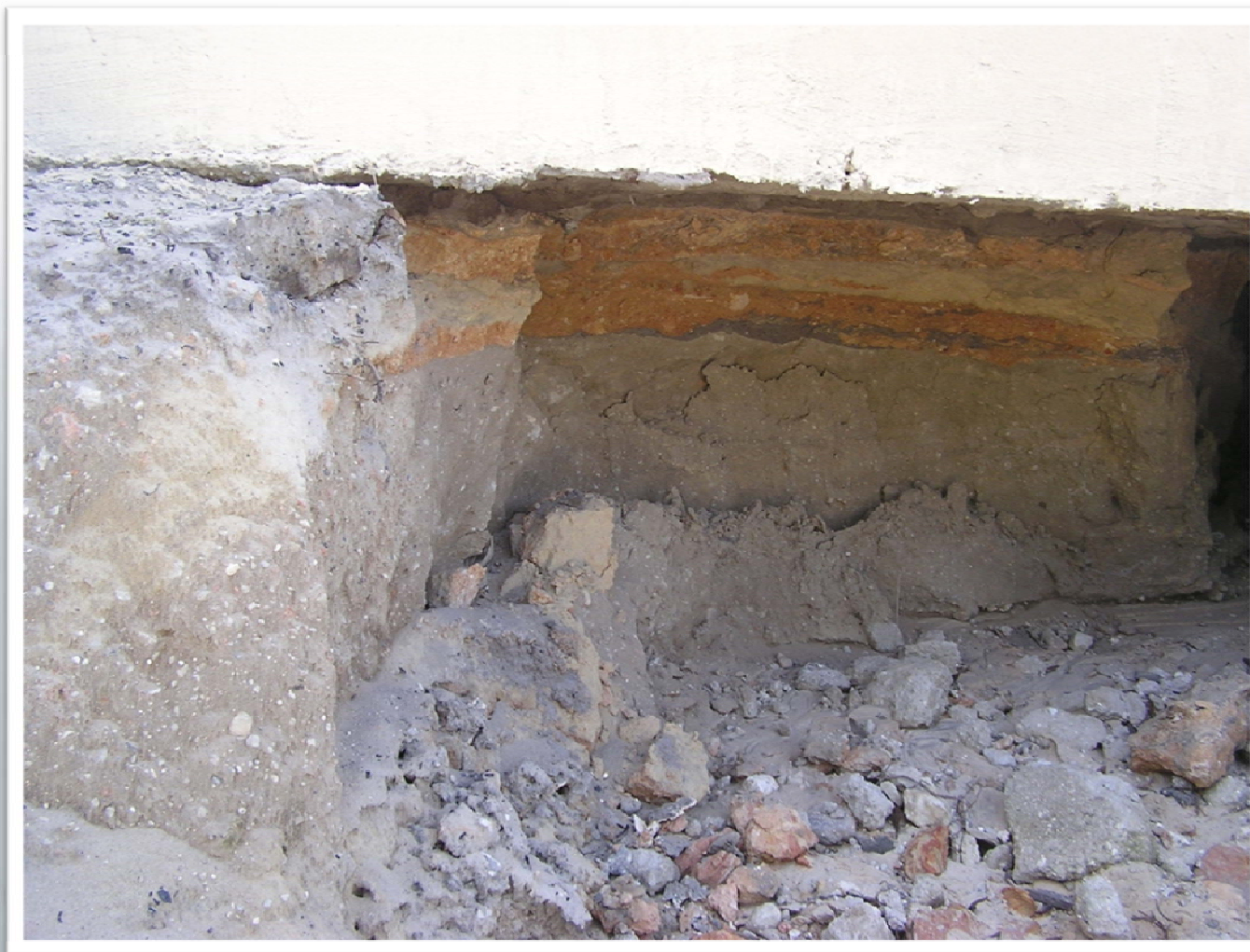
REUNION BRIDGE-Major Scour and Erosion of Approach Slab Resulting From Uncontrolled Surface Flow
