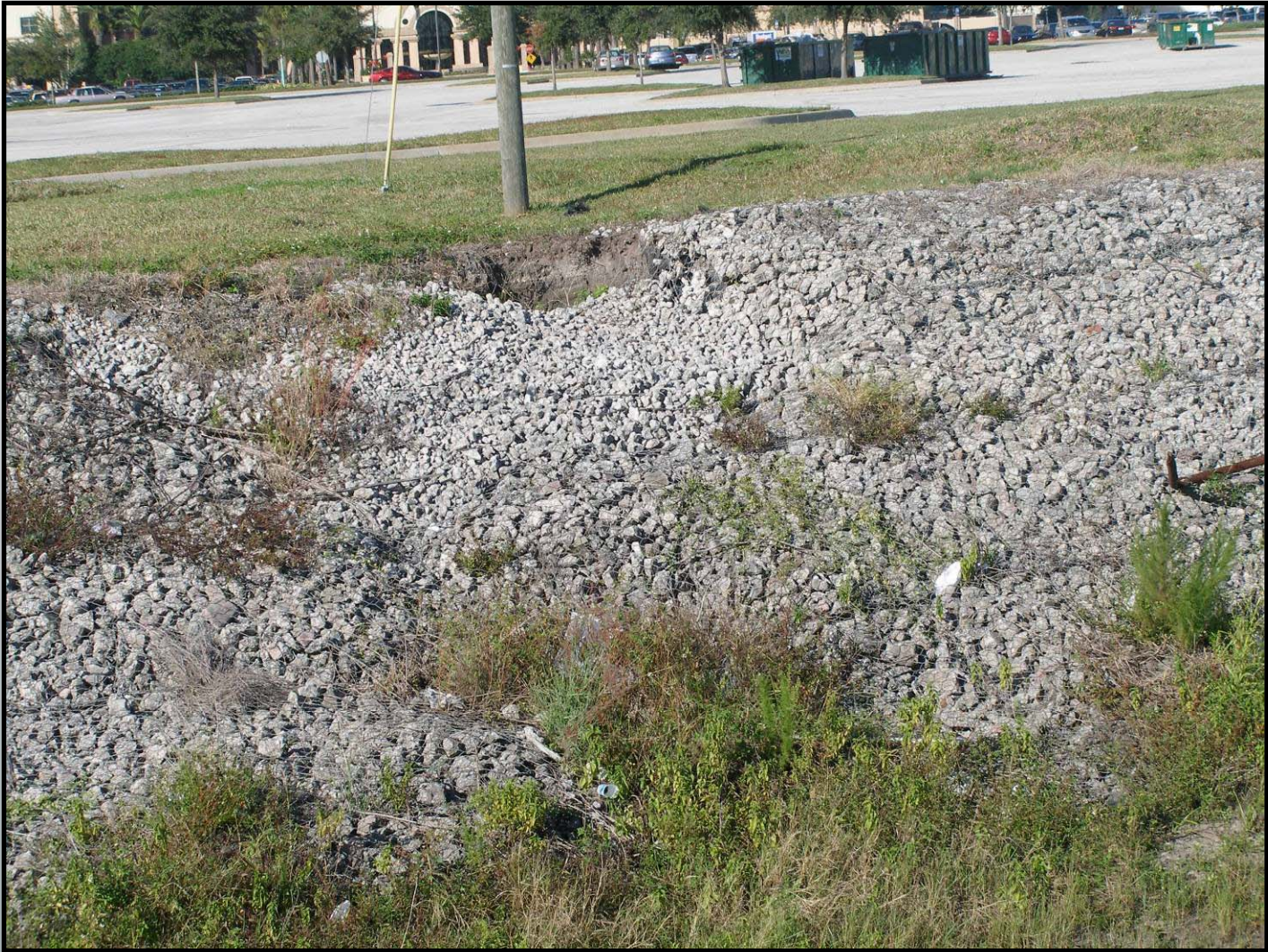
No anchorage of reno mattress on steep slope
