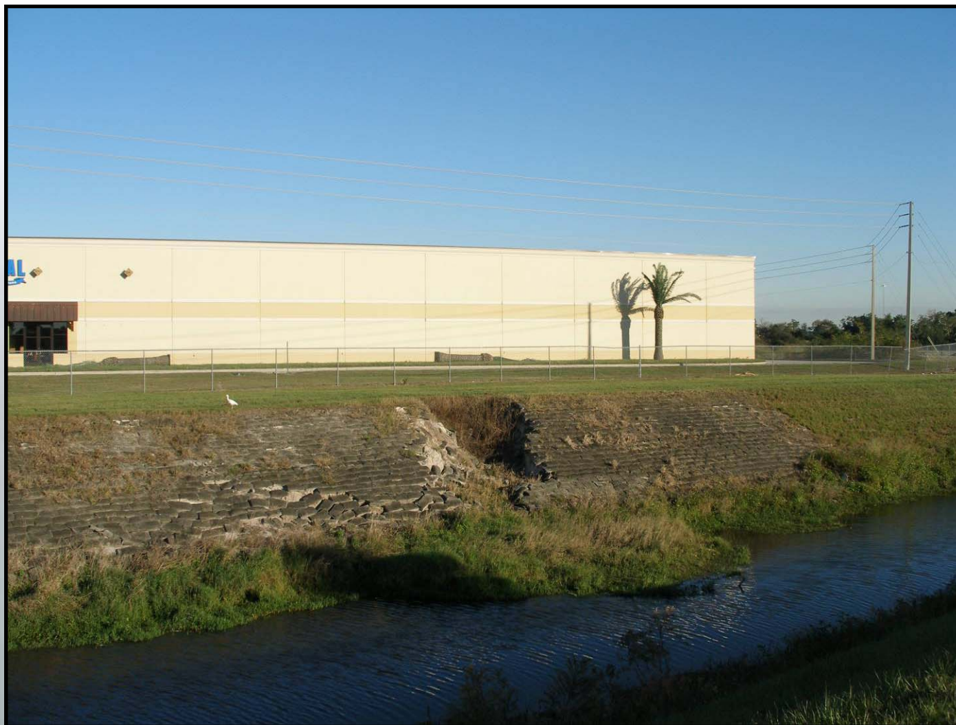
Slope erosion due to runoff
