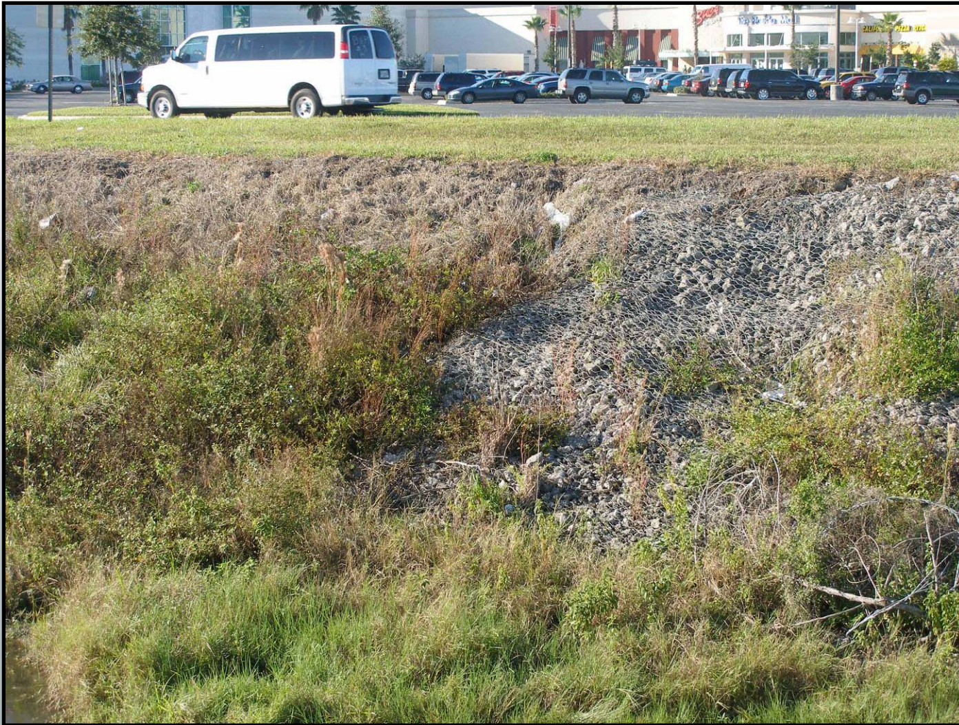
Slippage of reno mattress due to lack of anchorage on steep slope
