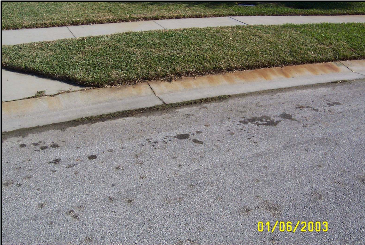
Leaching Over Curb
