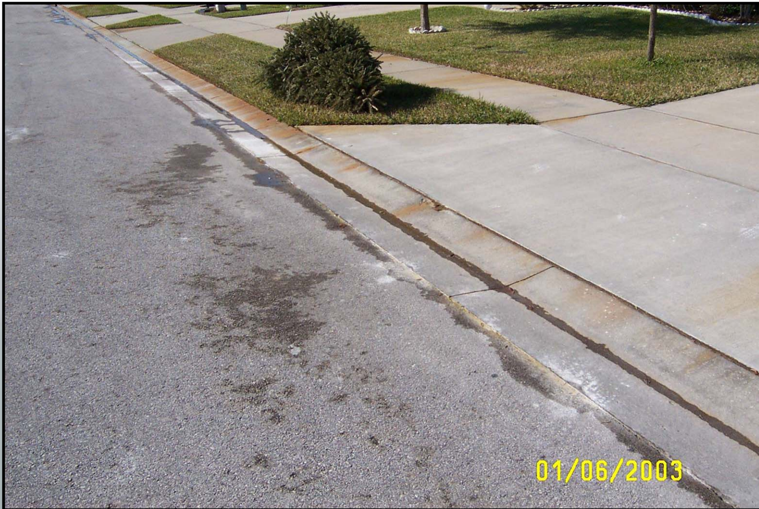
Leaching Over Curb
