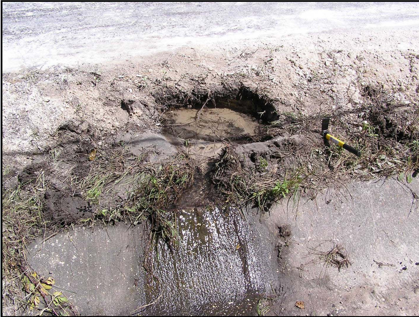
Seepage from Wolf Branch Road Subgrade, Just South of Cumulative Drainage Confluence Point
