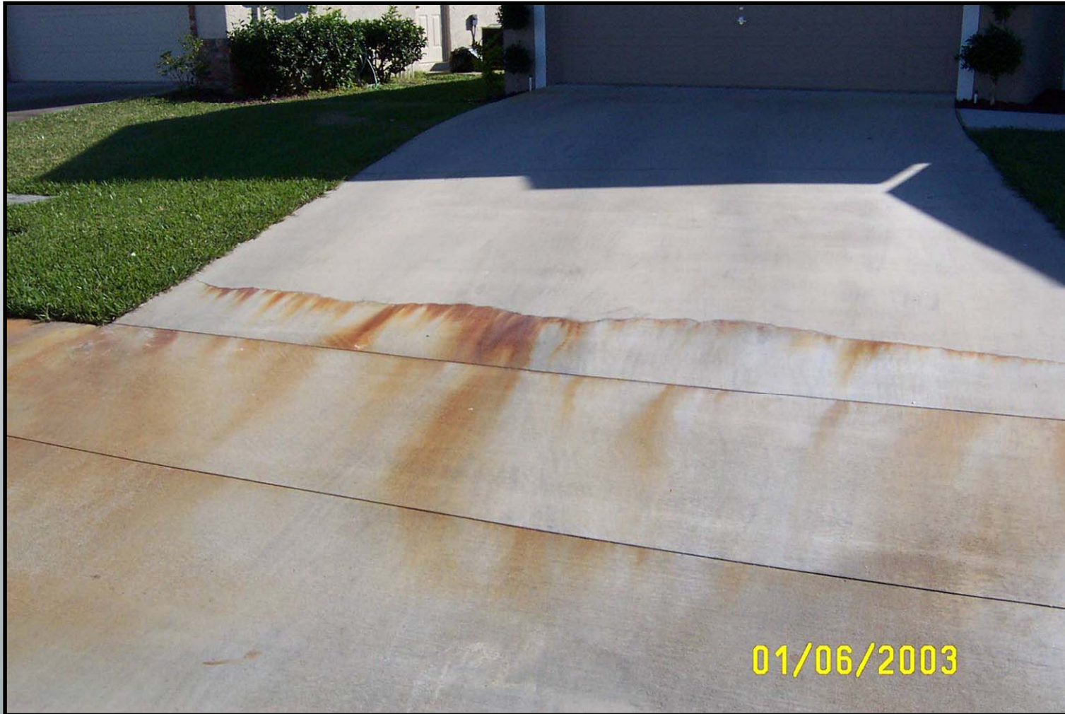
Leaching Over Curb
