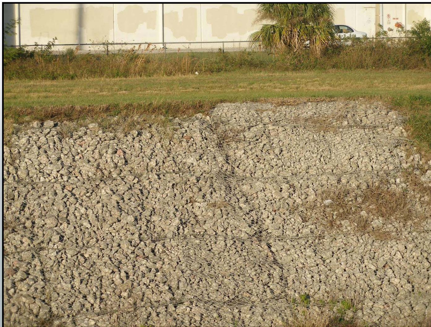
Slipping of reno mattress on steep canal slope
