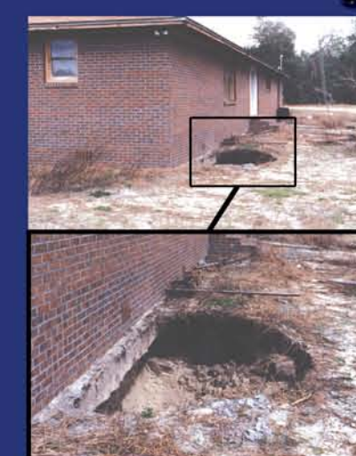
A collapse sinkhole in Wakulla County affecting a house foundation.
