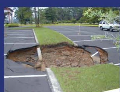
A collapse sinkhole in a church parking lot, northern Florida.
