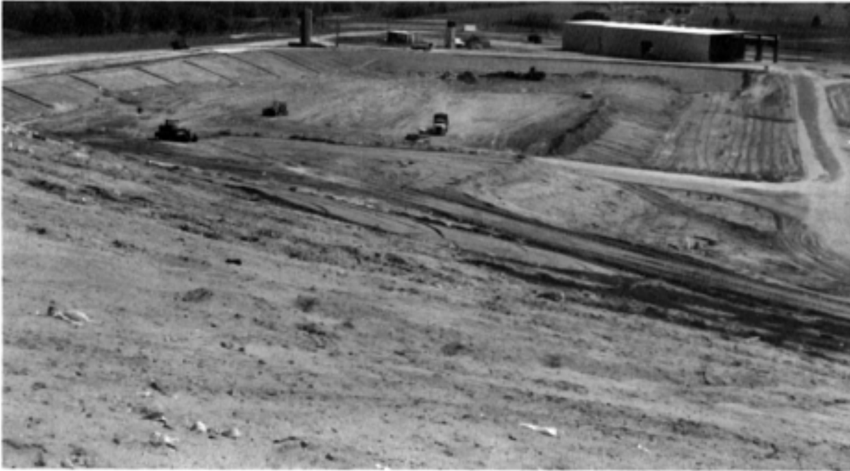
Figure 39. A new cell being prepared at the Marion County landfill, showing plastic liner on left and rear walls. The liner has been covered with sand on the other two walls for protection. Note the six leachate collection pipes on the left wall and the 30,000-gallon leachate holding tank in the left background (from Lane and Hoenstine, 1991).
