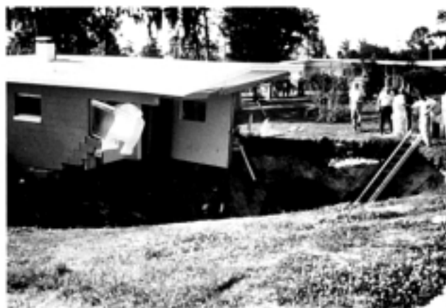
Sinkholes become a geologic hazard when they damage man's structures. FGS photograph.
