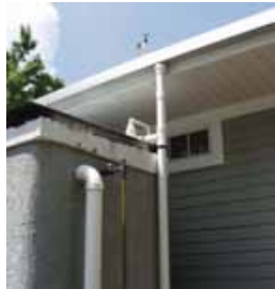
Cistern collects rain for nonpotable uses.
