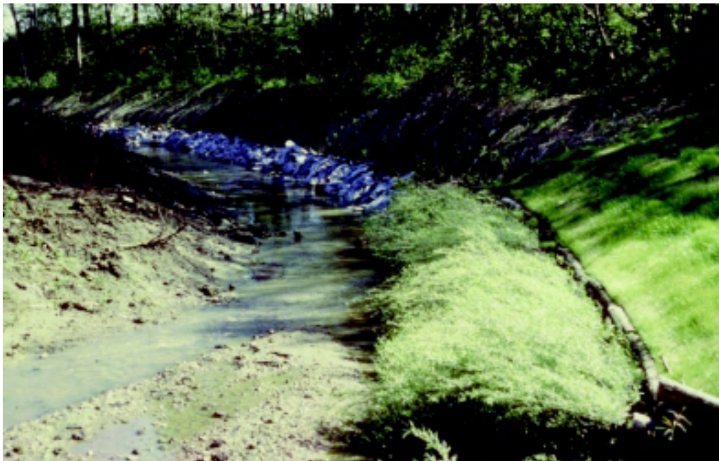
Figure 16-15c An established live cribwall system
